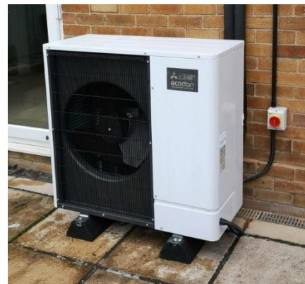
Air source heat pump condenser
