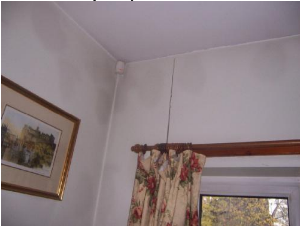
FIGURE 4 Internal damage to lounge
