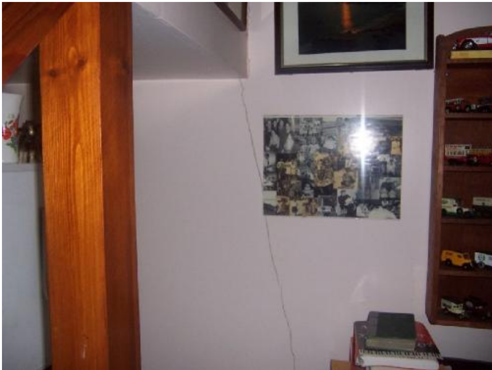
FIGURE 5 Internal damage to dining room
