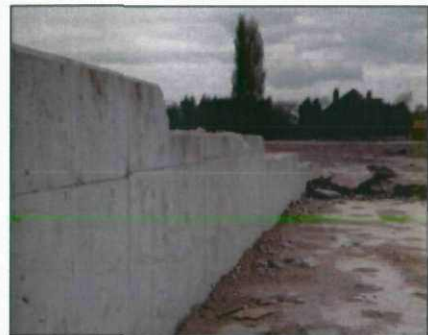
B sloping gradient to be constructed against wall, and top of wall to be taken down to below ground level
