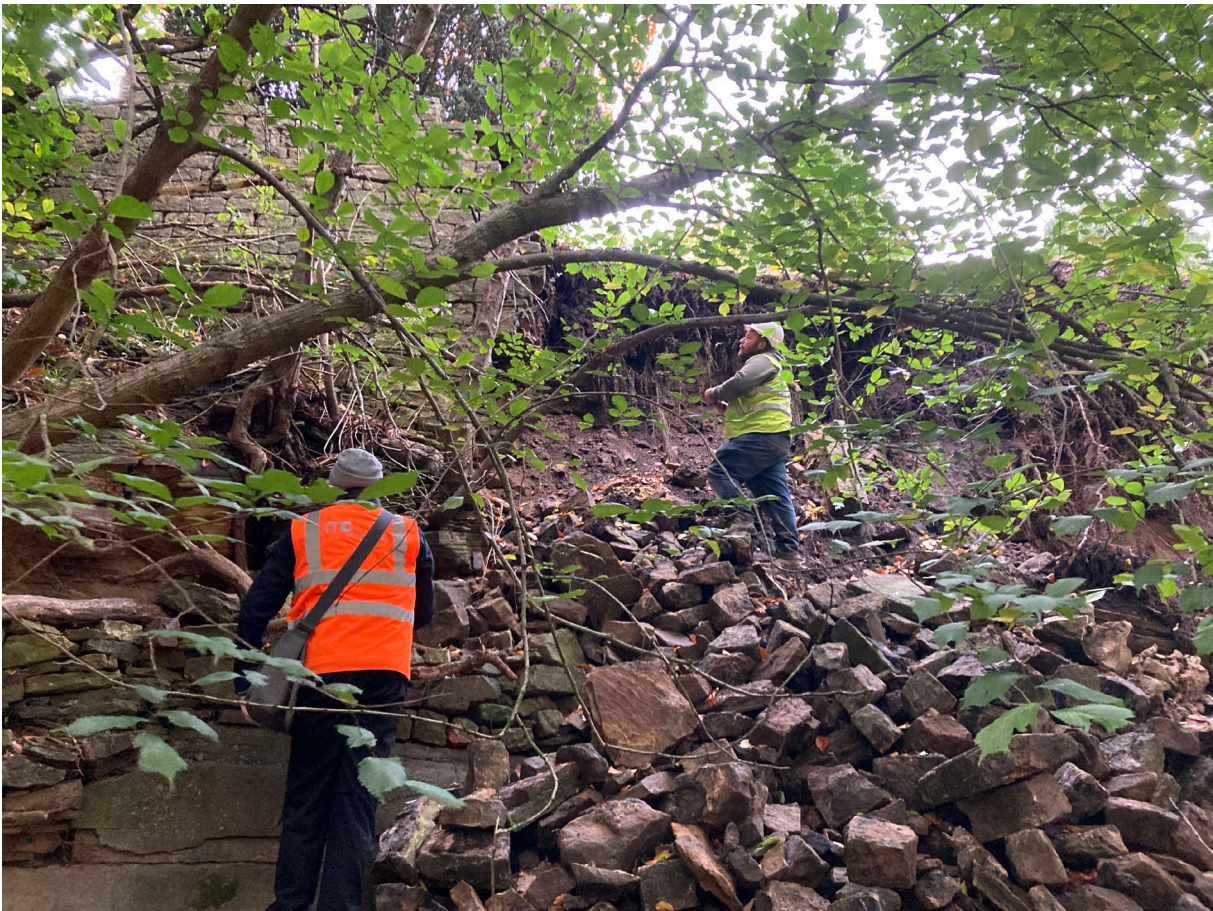
Collapsed section to Battlements
