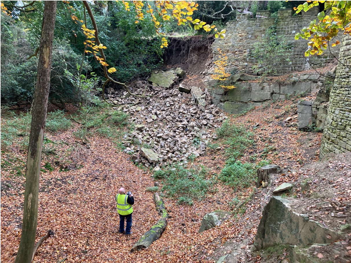
Collapsed section to Battlements
