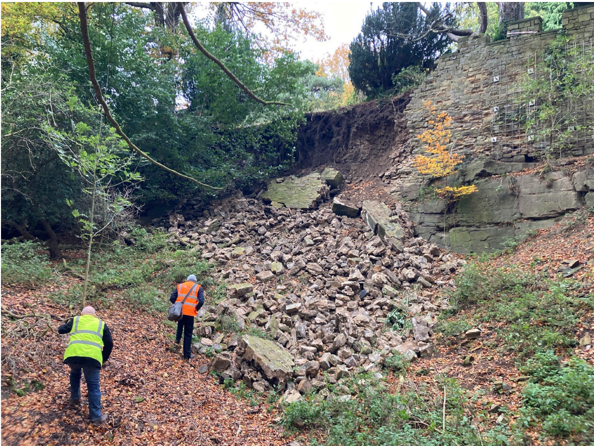
Collapsed section to Battlements
