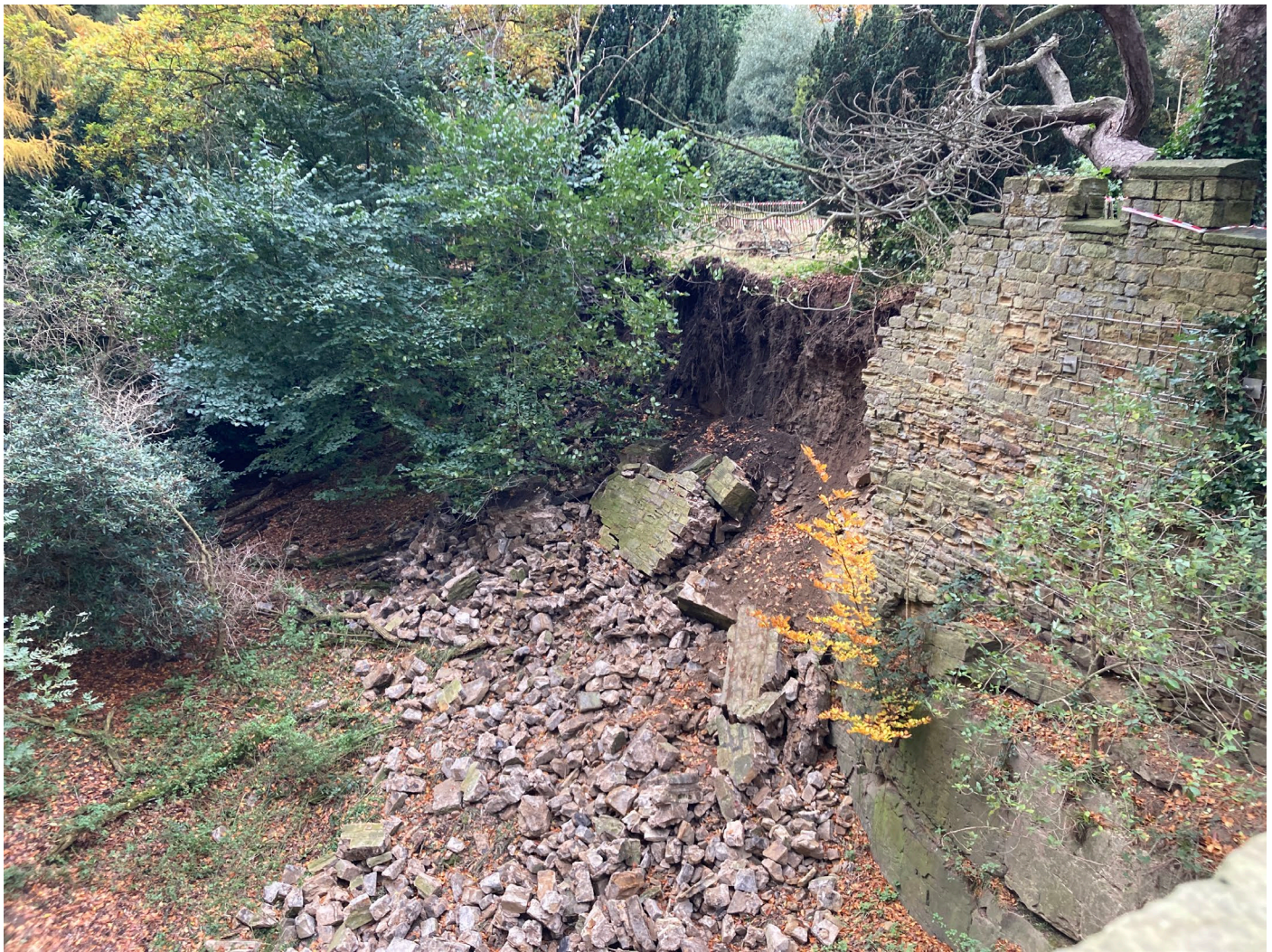
Collapsed section to Battlements
