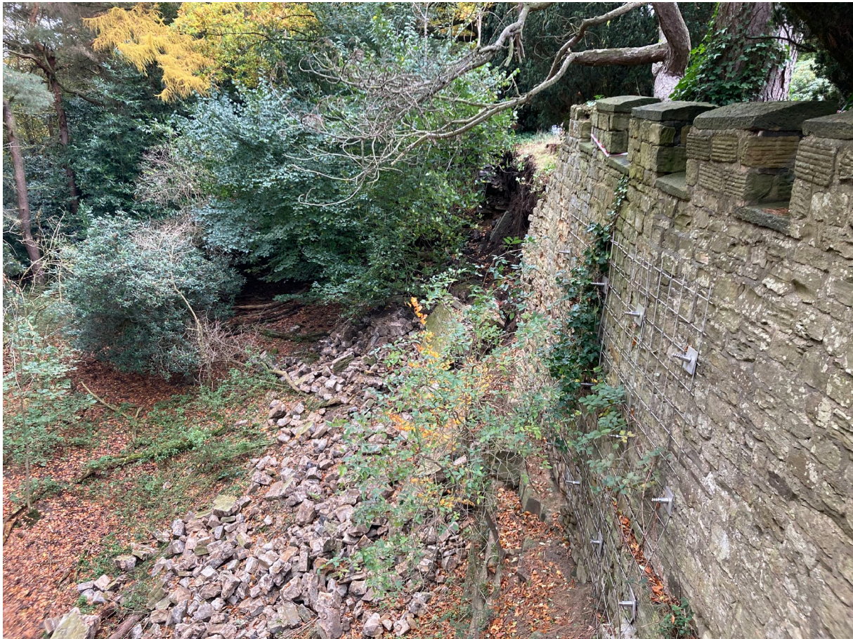
Collapsed section to Battlements adjacent to previous stainless steel pinning
