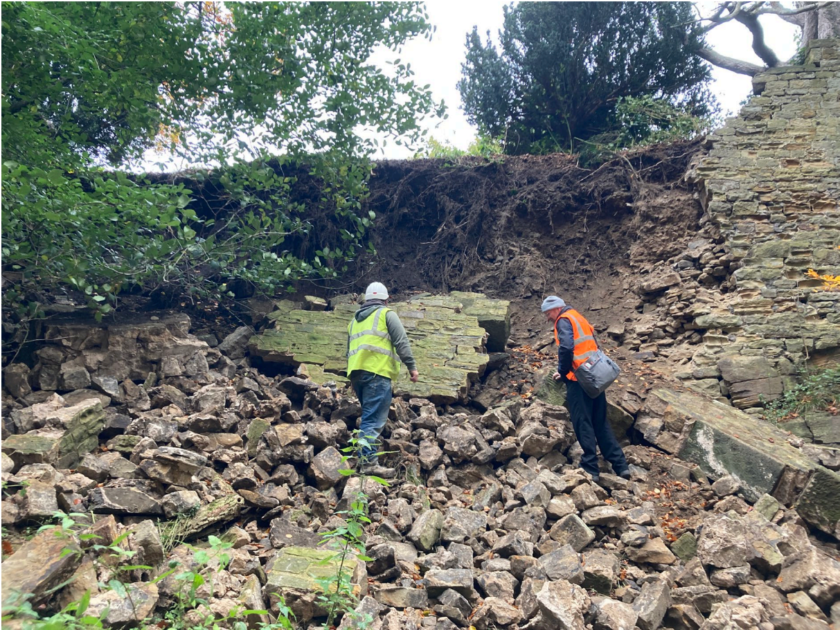
Collapsed section to Battlements
