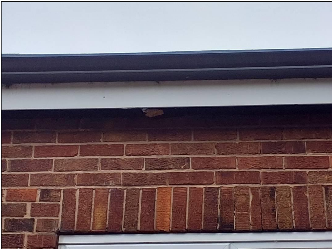
Photograph 9: Gap in soffit on B1
