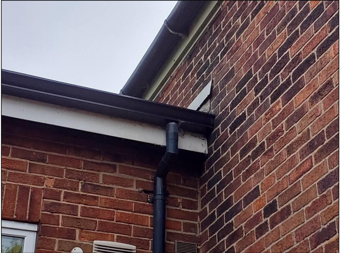
Photograph 8: Lifted flashing on B1
