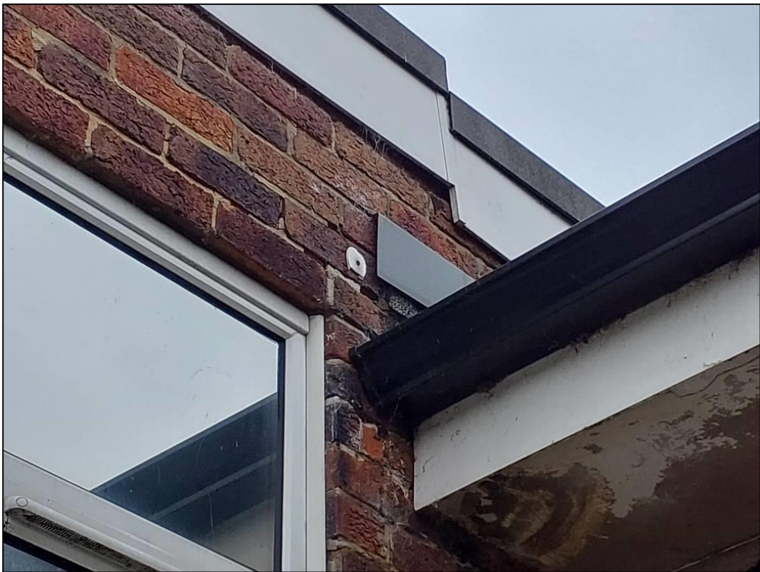
Photograph 10: Gaps under soffit on B1
