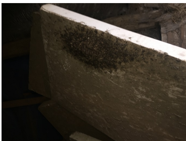
Plate 9 Aggregate of swallow droppings in Building 1
