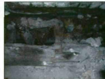
The Rotten Floor joists
