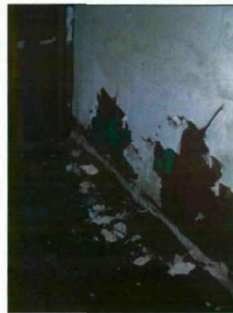
Dampness on the East Wall
