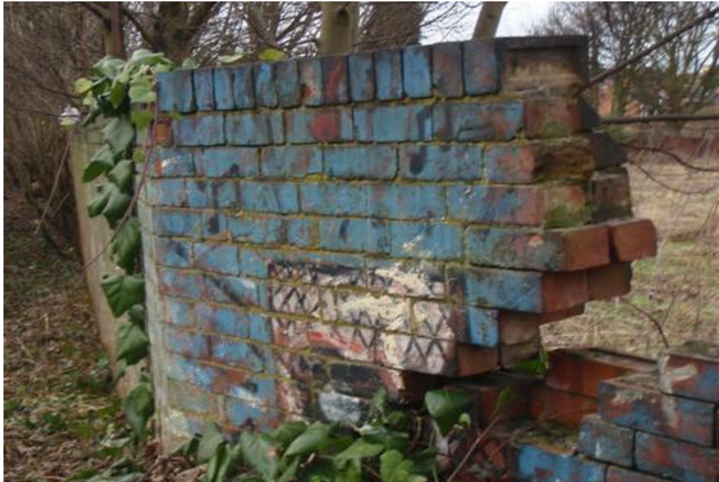
Photograph 3 Buckled free standing wall – middle and southern section (see figure 3)
