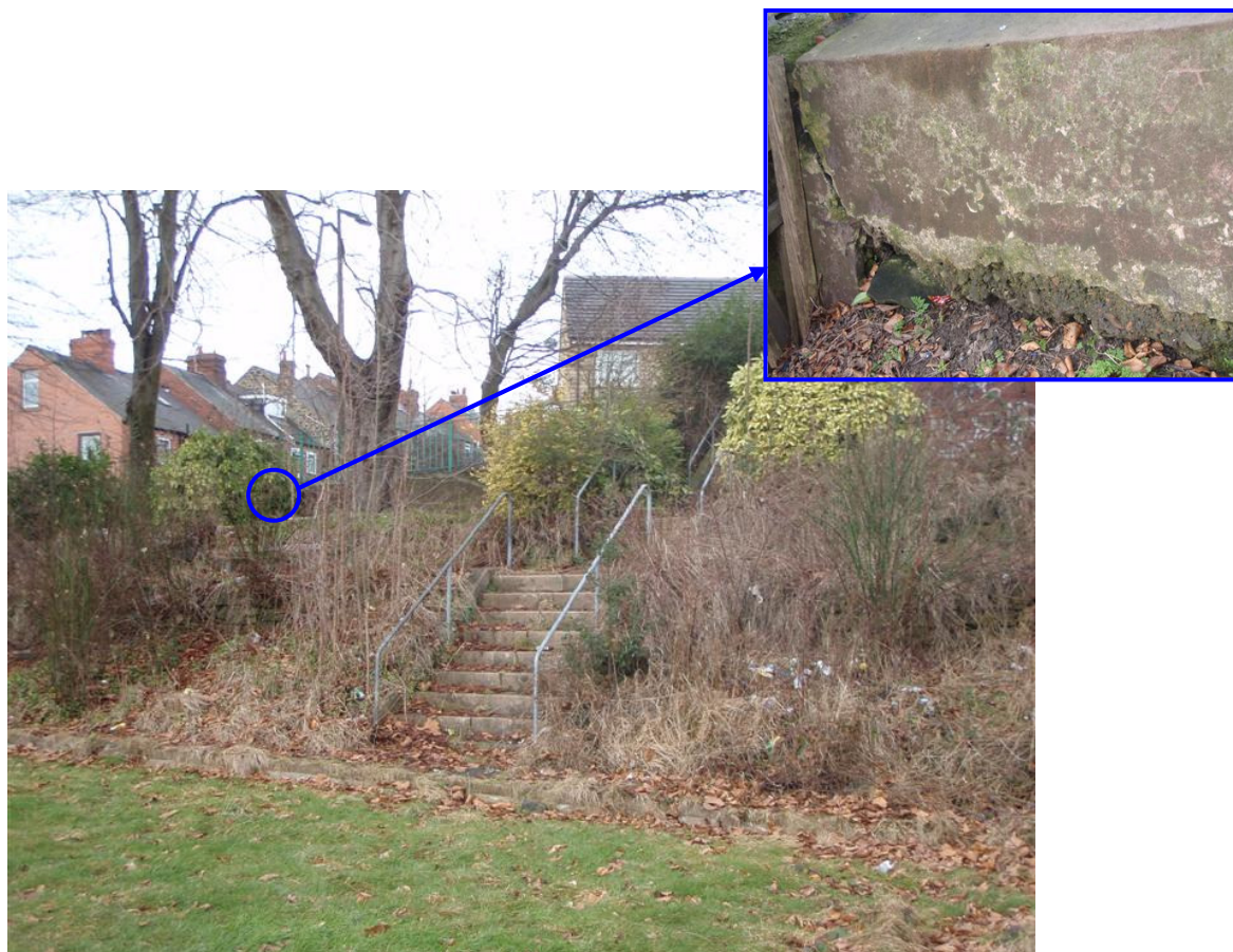
Photograph 2 Three tier retaining structure - with detail of cracking in concrete (see figure 3)
