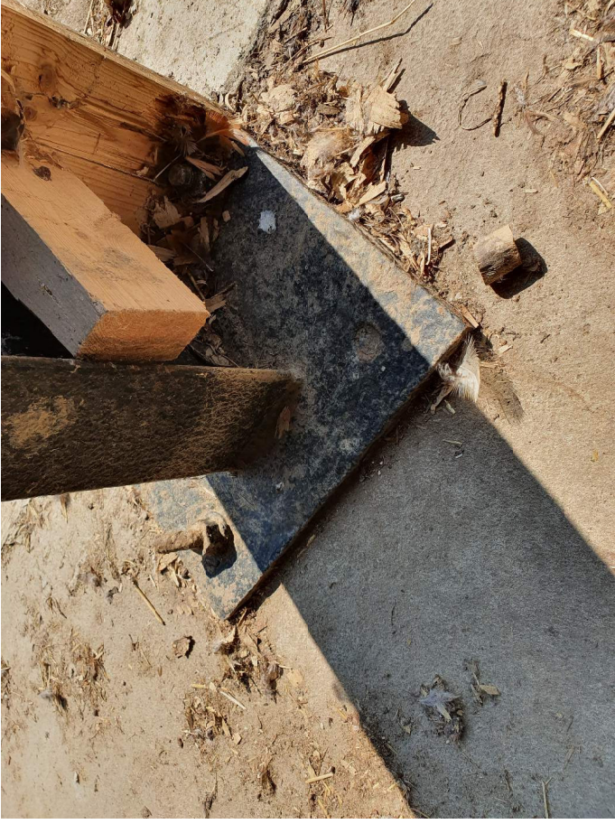
Bolt missing from column baseplate
