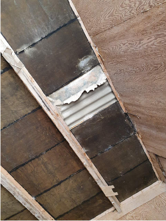
Missing soffit panel and damaged membrane
