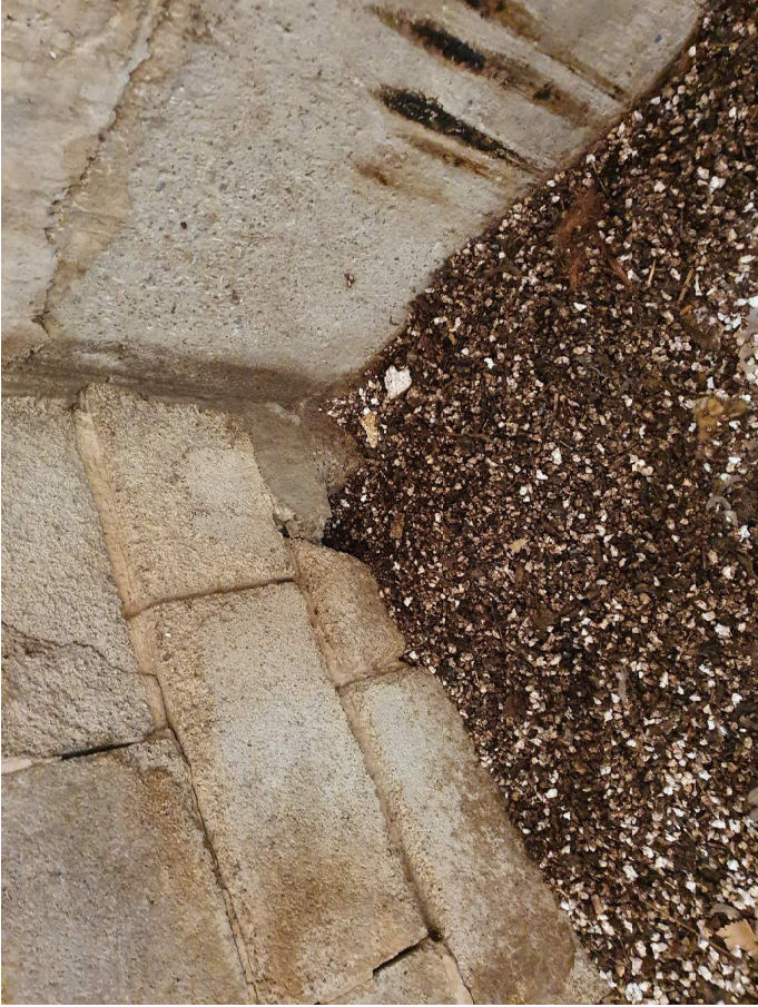
Fractured blockwork in northeast corner
