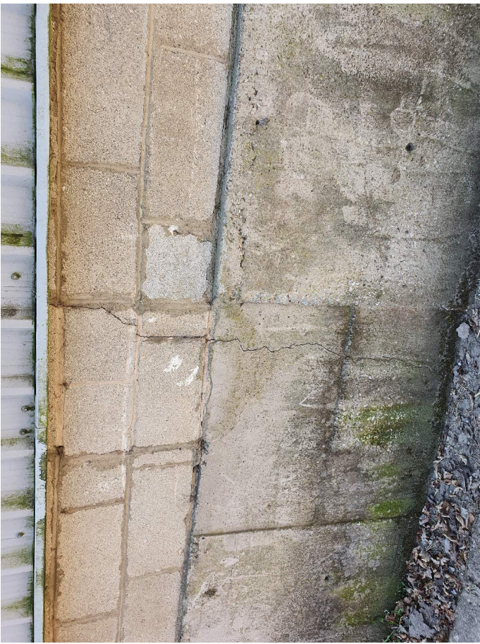
Cracked blockwork in east elevation
