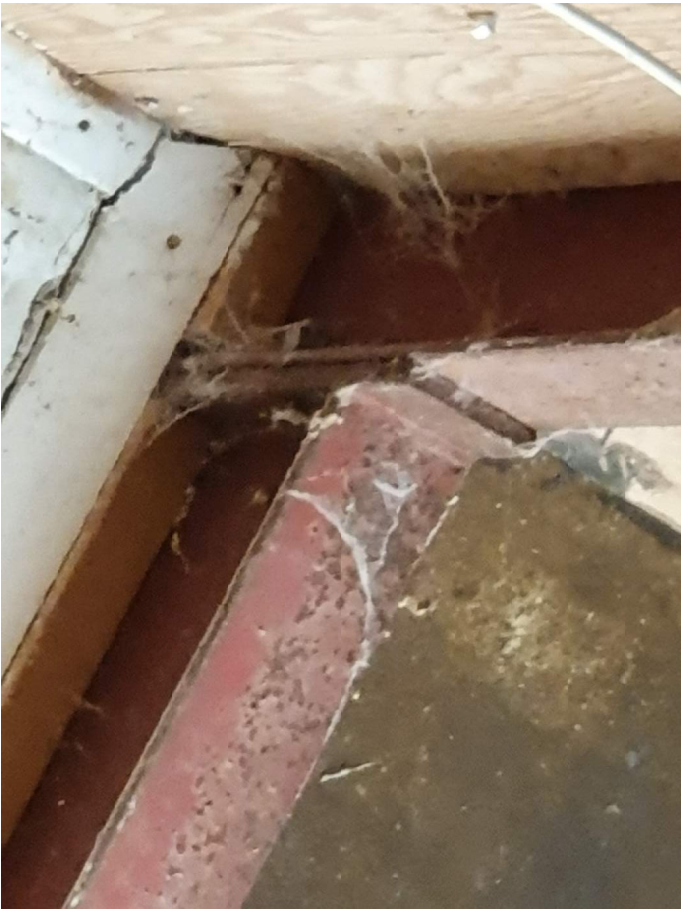
Mild rusting/pitting to steelwork
