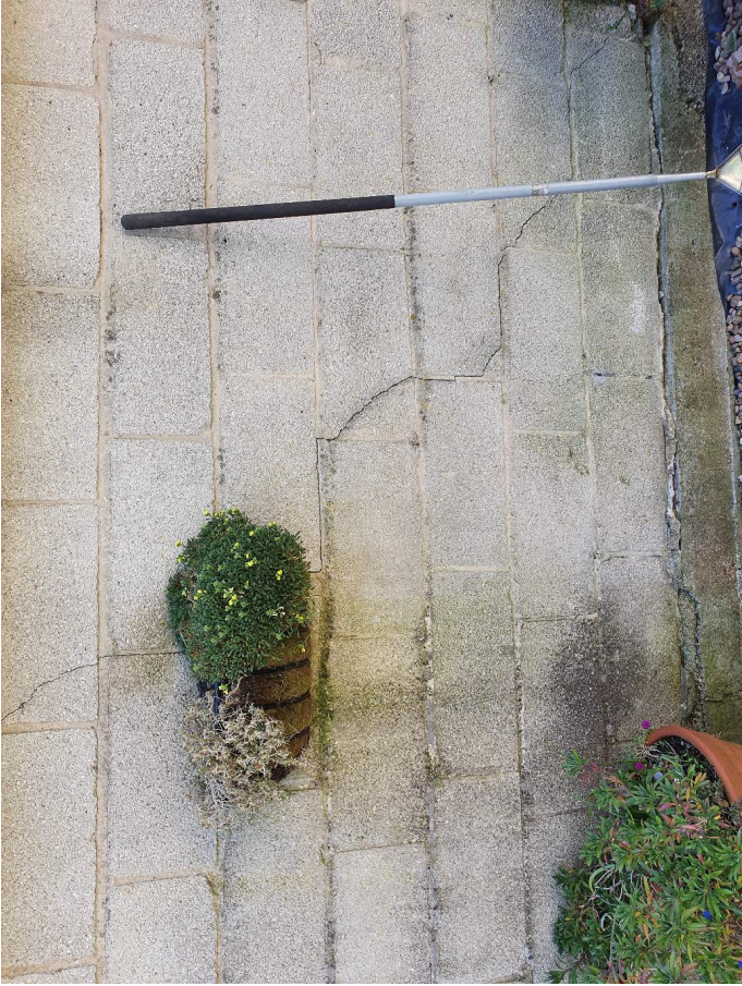
Cracked blockwork in north elevation
