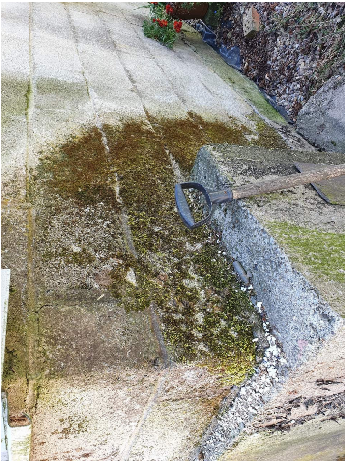
Evidence of long-term drainage issues
