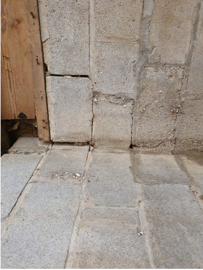
Cracked/displaced blocks in northeast corner
