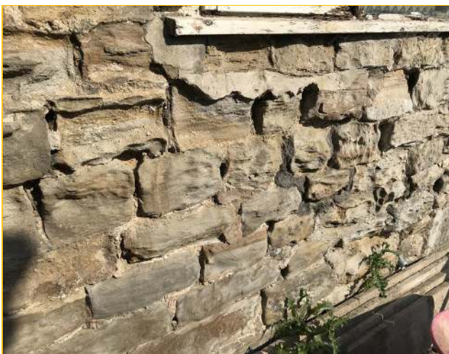
Photograph - 37 - Weathered masonry
