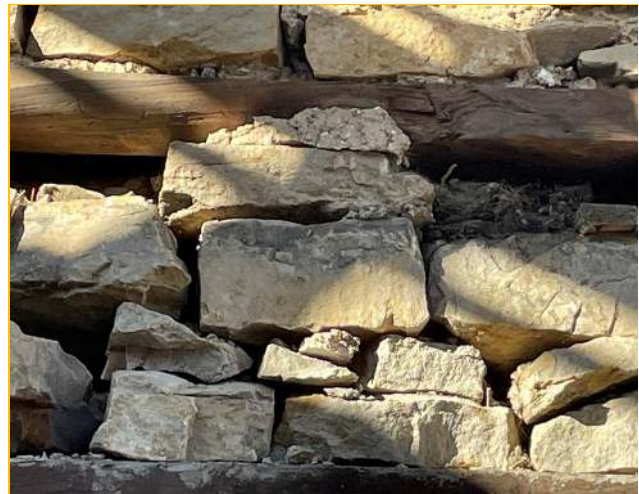
Photograph - 75 - Loss of mortar
