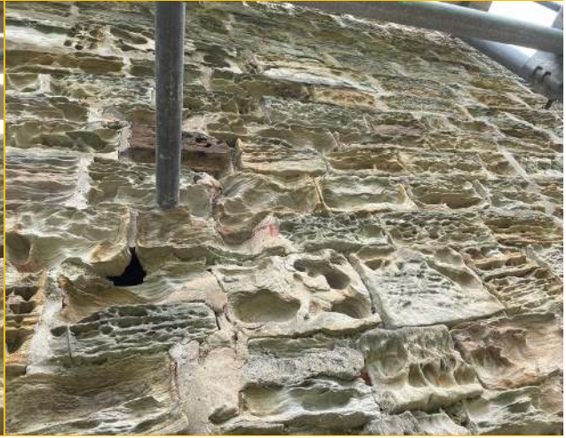
Photograph - 46 - Severe weathering
