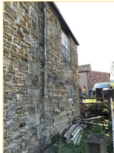
Photograph - 16 - Right extension right wall
