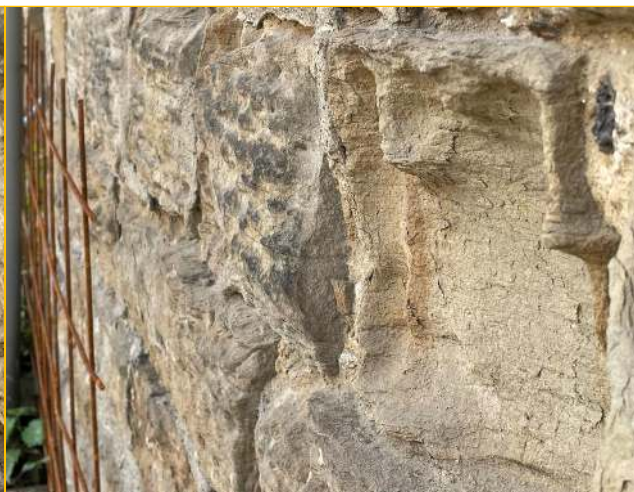
Photograph - 44 - Severe weathering
