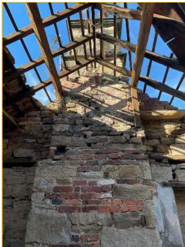
Photograph - 74 - Voiding to chimney breast
