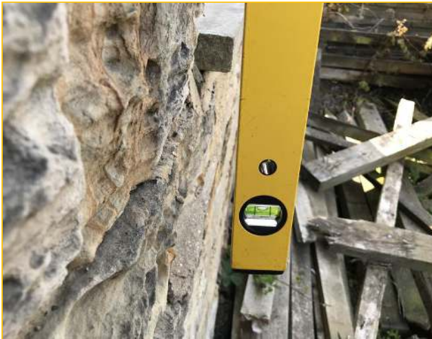
Photograph - 28 - Extent of tilt
