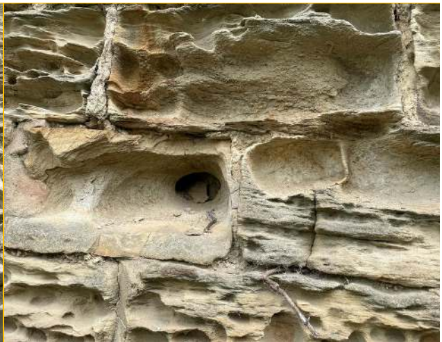
Photograph - 48 - Severe weathering
