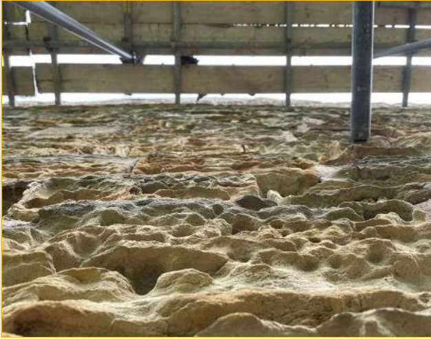
Photograph - 45 - Severe weathering
