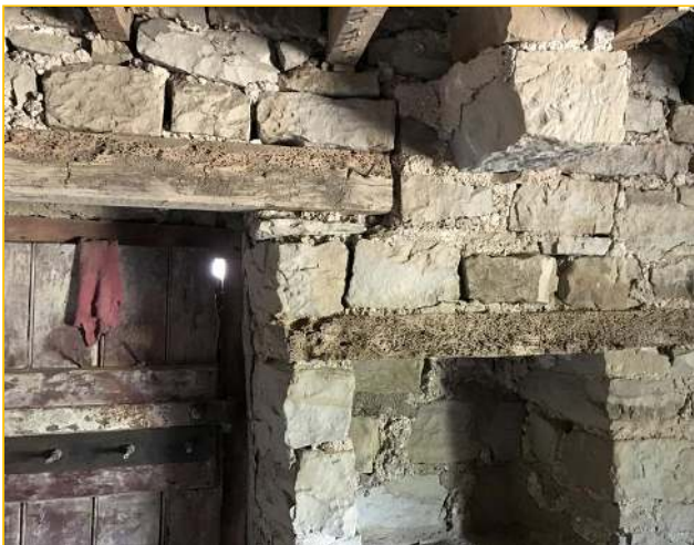
Photograph - 73 - Wood destroying insect damage
