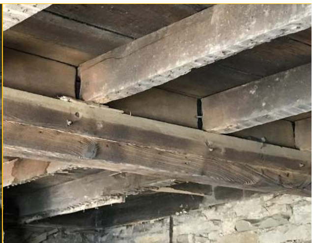
Photograph - 55 - Limited bearing
