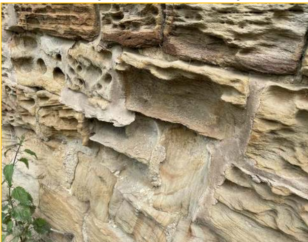
Photograph - 49 - Severe weathering
