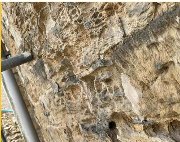
Photograph - 43 - Severe weathering
