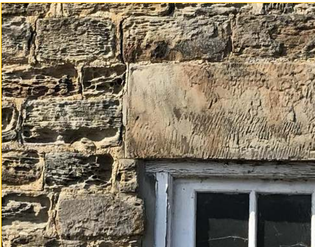
Photograph - 31 - Limited bearing
