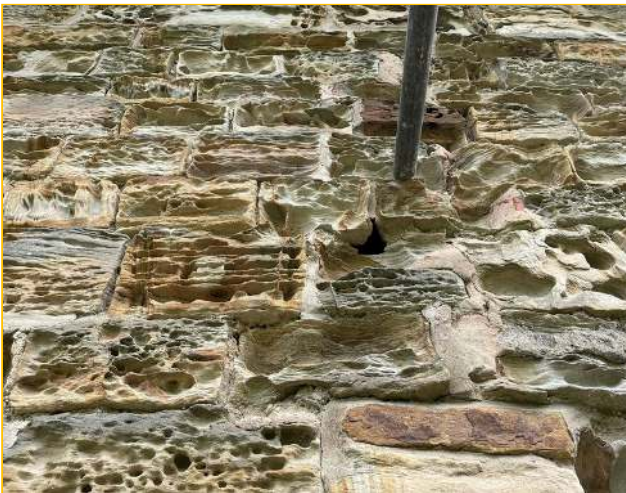
Photograph - 47 - Severe weathering
