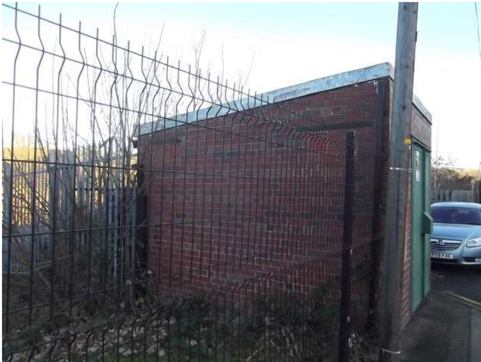
Plate 4. The Electrical substation in the south west corner of the site.
