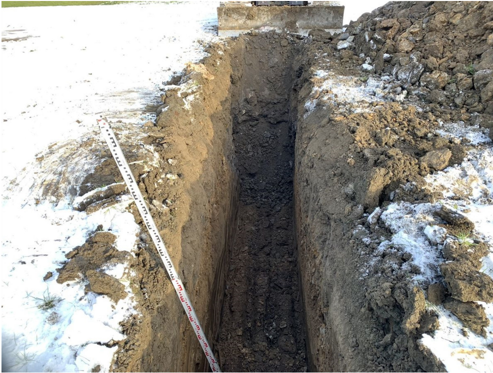
Photograph 28: Trial pit TP04. Eastern face of trial pit, view from the west to the east.
