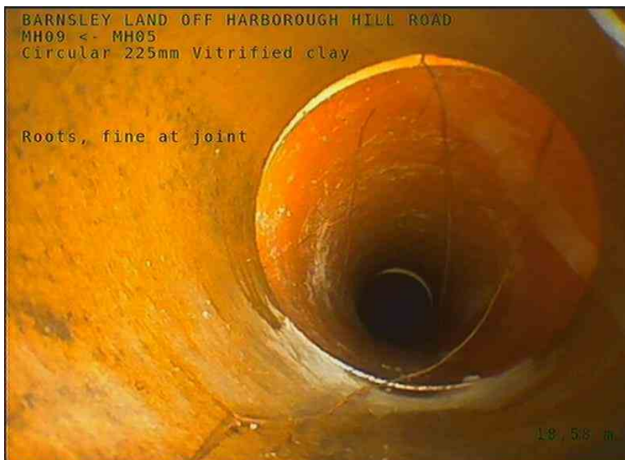
8, 00:02:58, 18.58 m Roots, fine at joint, CIP PATCH REQ
