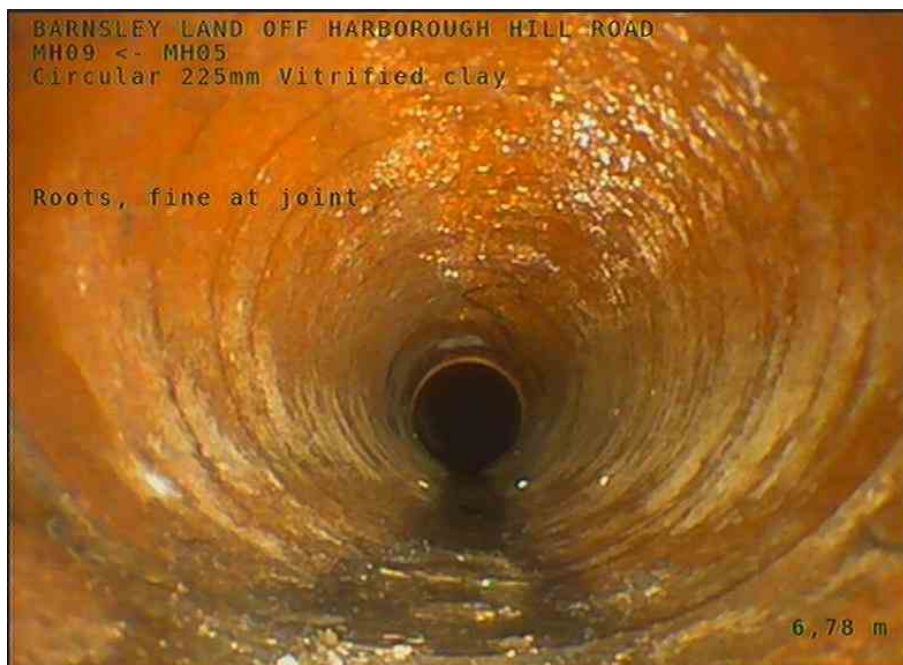
4, 00:01:21, 6.78 m Roots, fine at joint, CIP PATCH REQ
