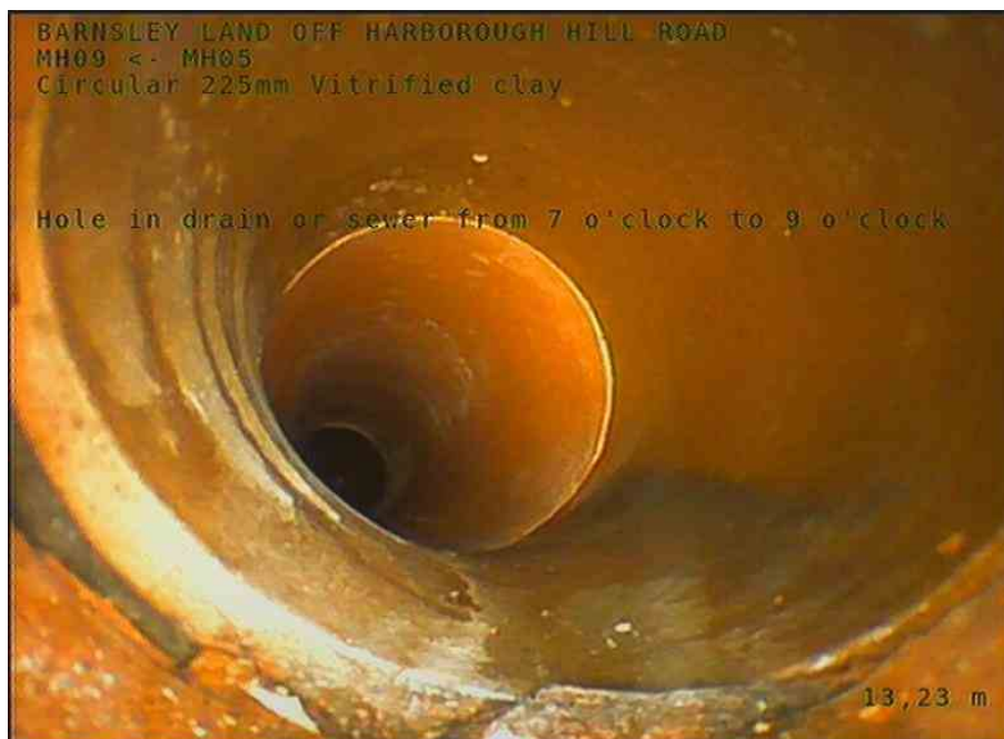
6, 00:02:19, 13.23 m Hole in drain or sewer from 7 o'clock to 9 o'clock, CIP PATCH
