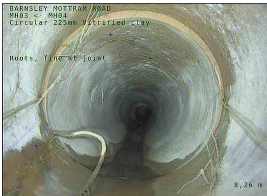
2, 00:00:50, 8.26 m Roots, fine at joint, CIP PATCH REQ
