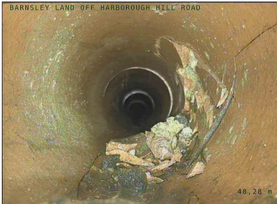
3, 00:04:43, 48.28 m Broken pipe from 1 o'clock to 6 o'clock
