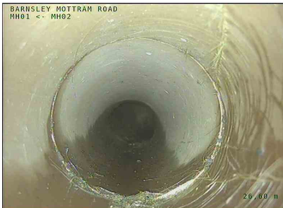
2, 00:03:01, 26.60 m Roots, fine at joint, CIP PATCH REQ
