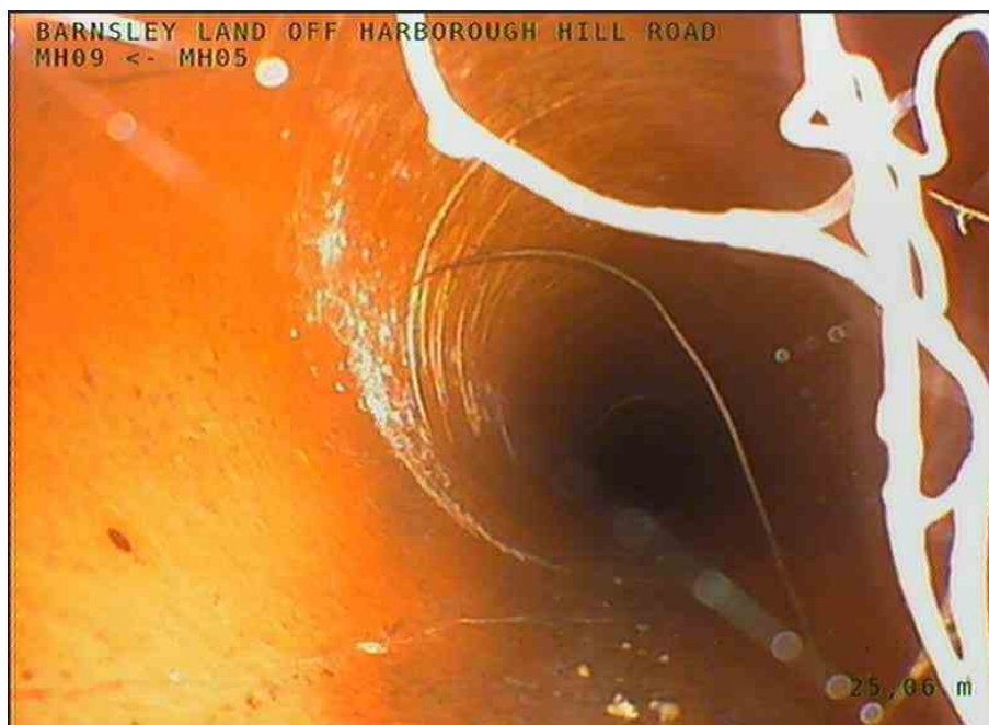
10, 00:04:15, 25.06 m Roots, fine at joint, CIP PATCH REQ
