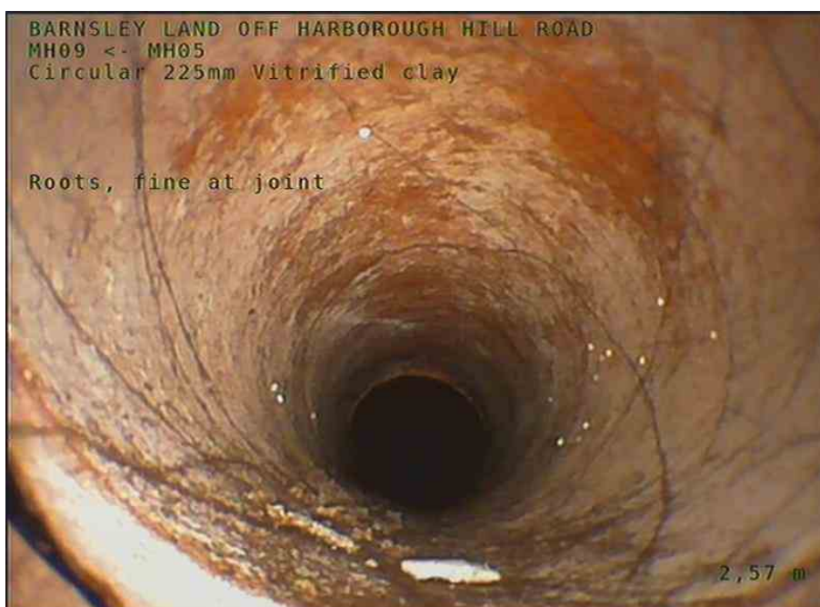
2, 00:00:40, 2.57 m Roots, fine at joint, CIP PATCH REQ
