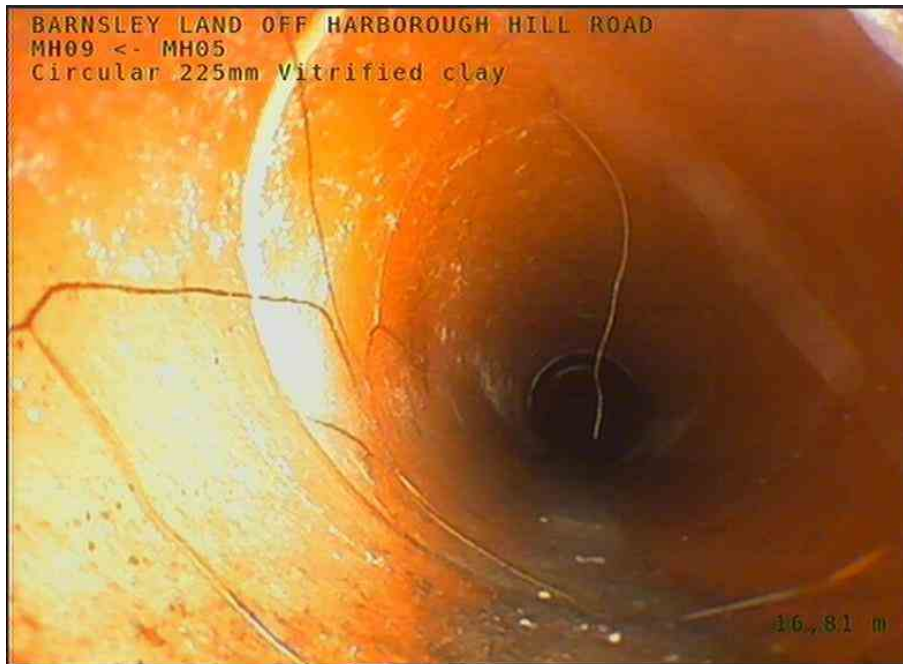
7, 00:02:43, 16.81 m Roots, fine at joint, CIP PATCH
