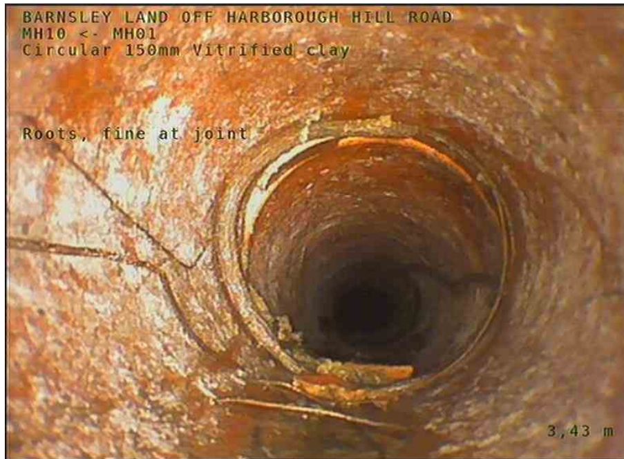
1, 00:01:09, 3.43 m Roots, fine at joint, CIP PATCH REQ
