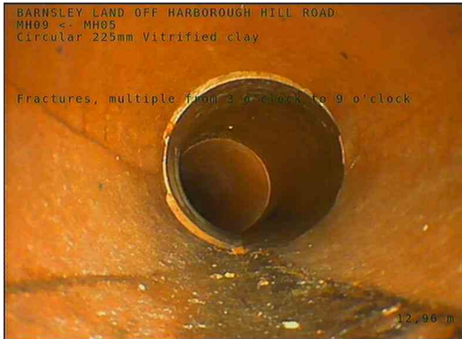
5, 00:02:01, 12.96 m Fractures, multiple from 3 o'clock to 9 o'clock, CIP PATCH REQ
