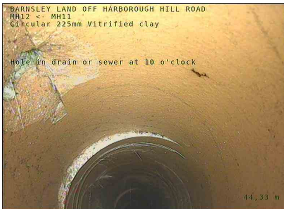
2, 00:02:57, 44.33 m Hole in drain or sewer at 10 o'clock
