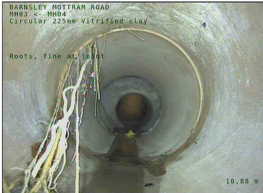
3, 00:01:05, 10.88 m Roots, fine at joint, CIP PATCH REQ
