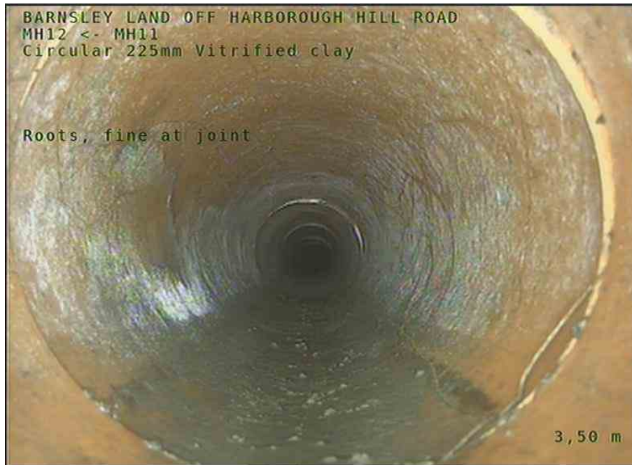
1, 00:00:26, 3.50 m Roots, fine at joint, CIP PATCH REQ
