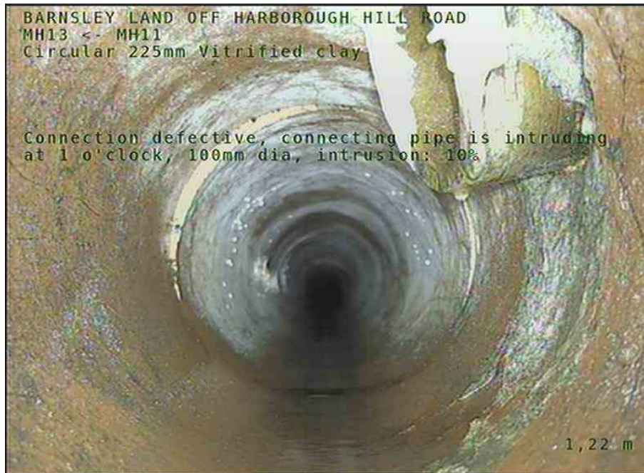
1, 00:00:21, 1.22 m Connection defective, connecting pipe is intruding at 1 o'clock, 100mm dia, intrusion: 10%
