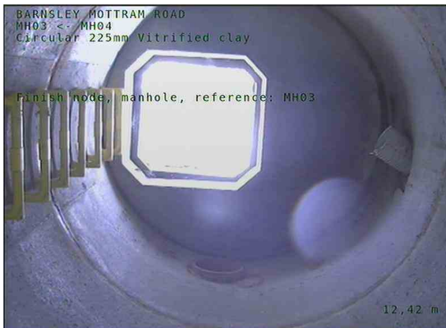
4, 00:01:29, 12.42 m Finish node, manhole, reference: MH03, NO COVER ON MANHOLE
