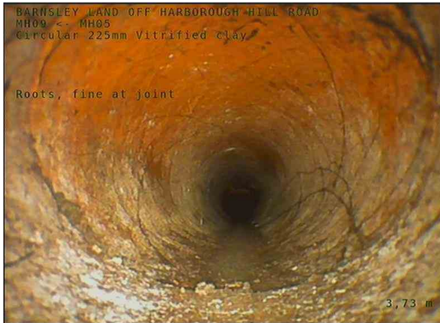
3, 00:00:57, 3.73 m Roots, fine at joint, CIP PATCH REQ
