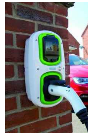
Typical Wall Mounted Electric Vehicle Charging Point
