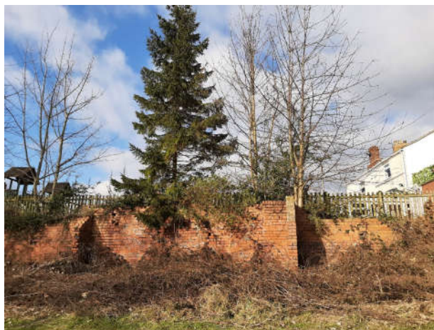
Photo 3: Trees situated in the retaining wall at the northern boundary
