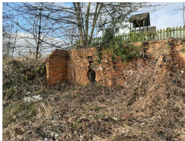
Photo 4: Damage to the retaining wall, which may be exacerbated by further tree growth
