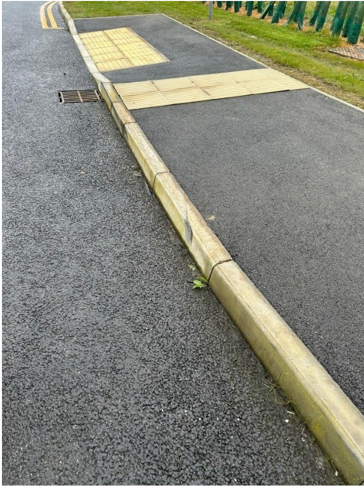
Image 15 – Damaged kerbs at joints and tyre scrub
