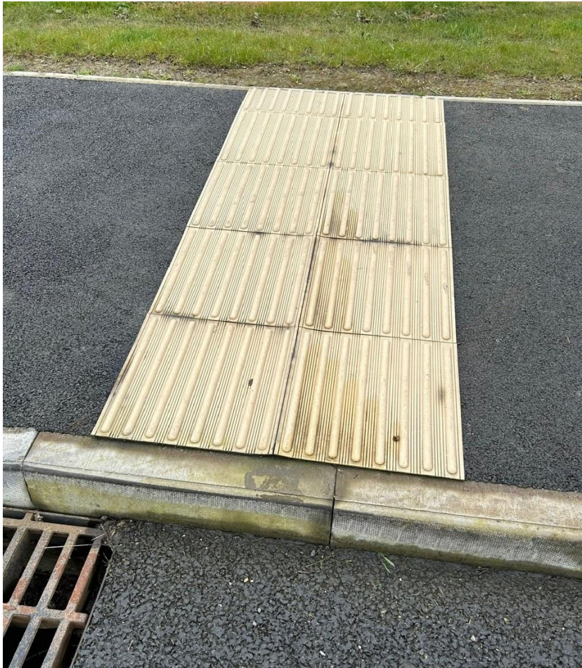
Image 16 – Corduroy warning surface lifting
