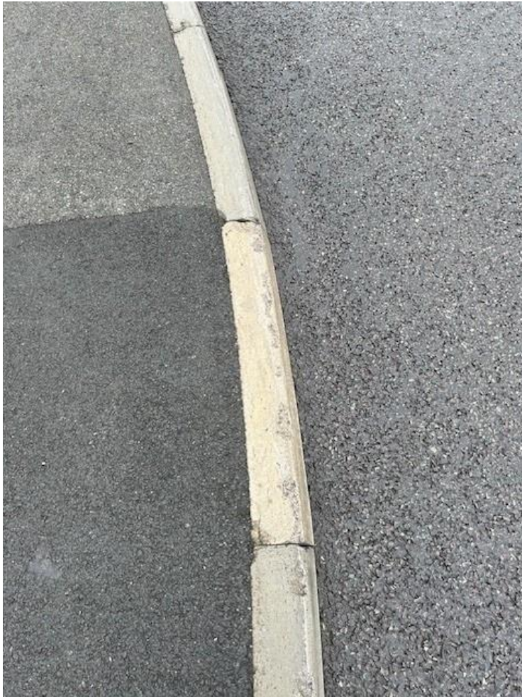
Item 7 – Damaged radius kerb
