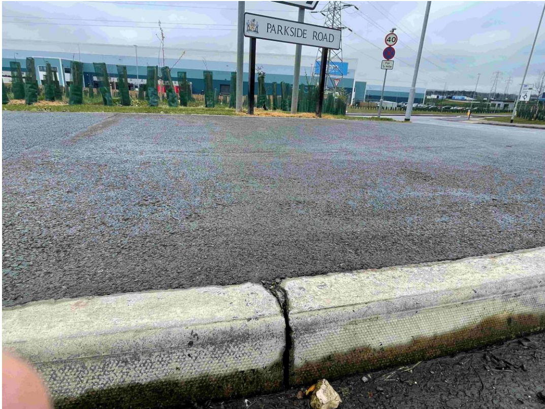
Image 14 – Chipped kerb at joint
