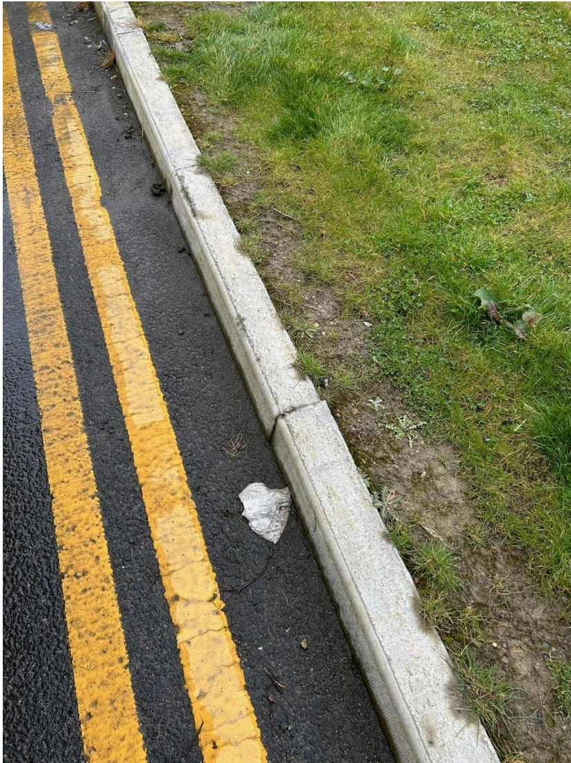
Image 18 – Kerb out of line
