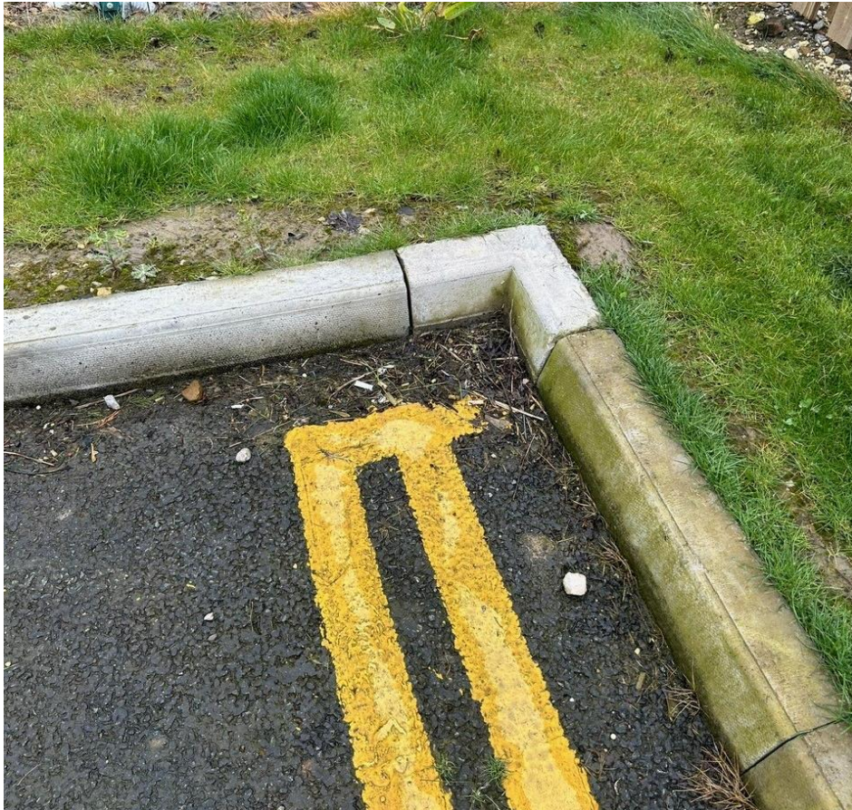
Image 21- Damage to corner kerb
