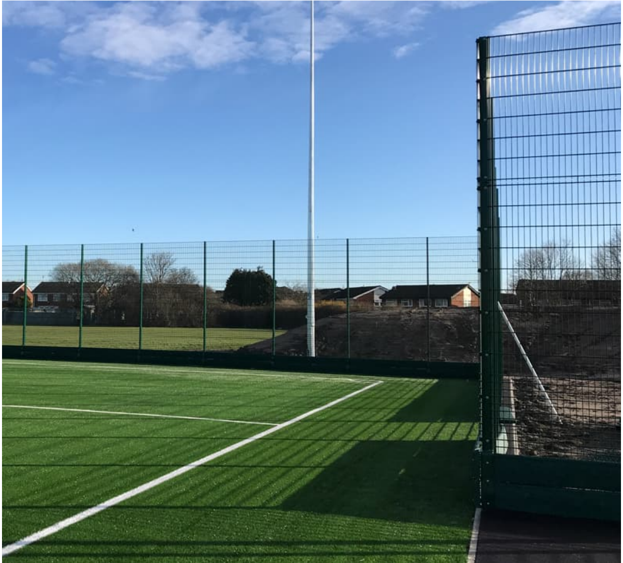
Example photograph of 4.5m high perimeter fencing
