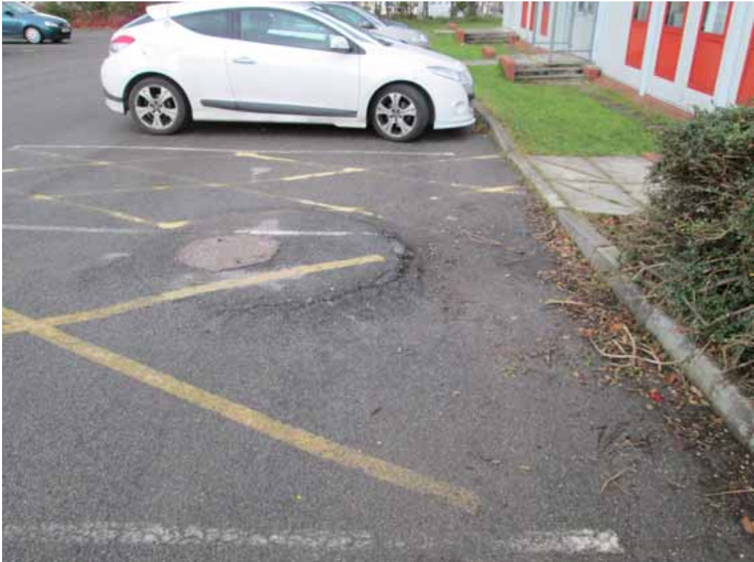
Photo 10 – Evidence of settlement of car parking surfacing
