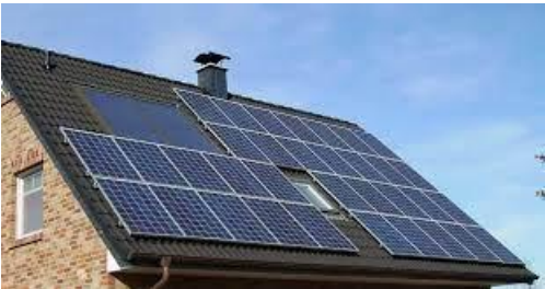
Photovoltaic Solar Panels fitted to roof
