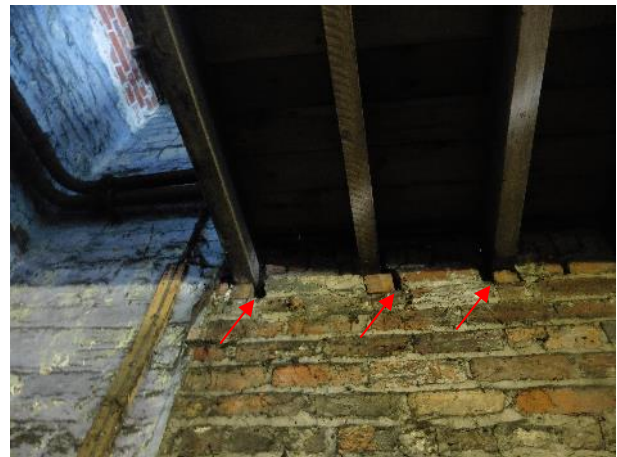
Gaps around joists filled with cobwebs
