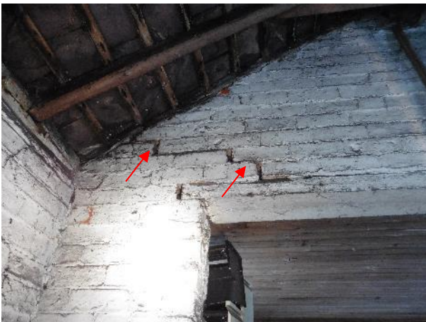
Cracks in brickwork filled with cobwebs
