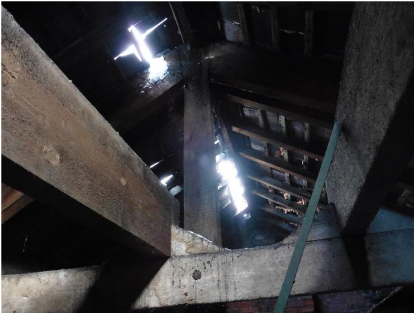
Large holes in roof allowing light and water into void
