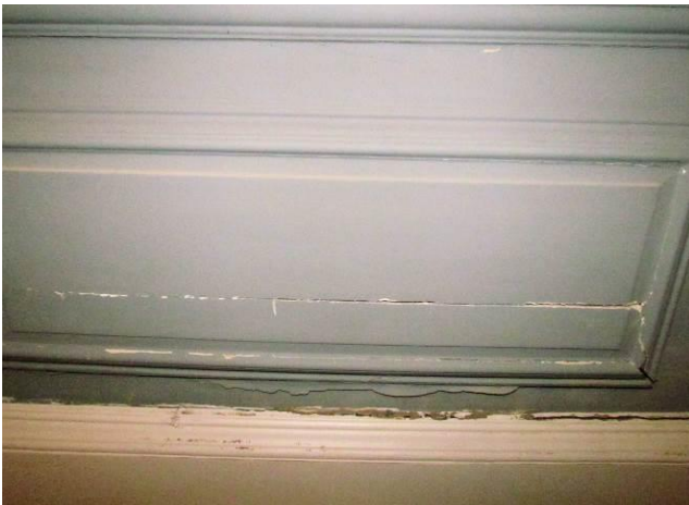
Cracks in Panel Below Opening
