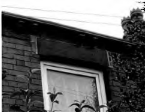
Photo 11: Central Window Gaps in Repointing adjacent to Lintel
