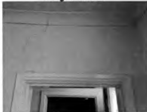
Photo 34: LHS Reception 2 mm Cracking over Front Doorway
