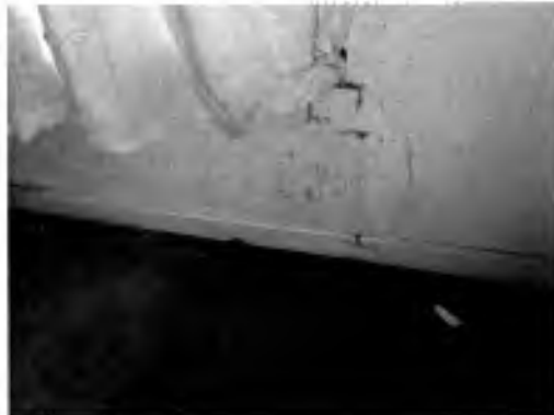
Photo 44: Rear Bedroom 1.5 mm Cracking below Window
