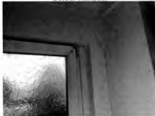
Photo 46: 2 mm Rear Bathroom Window
