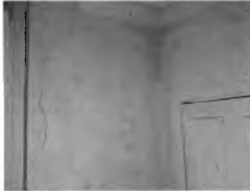
Photo 32: Cracking to 1.5 mm in Front Lounge near Door
