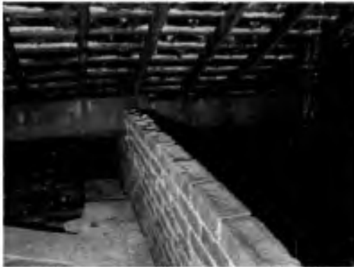
Photo 55: Central Supporting Pier Purlin Rotation
