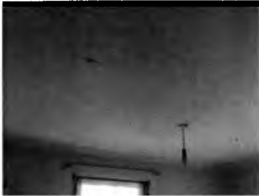
Photo 49: LHS Front Bedroom Cracking to 1.0 mm.
