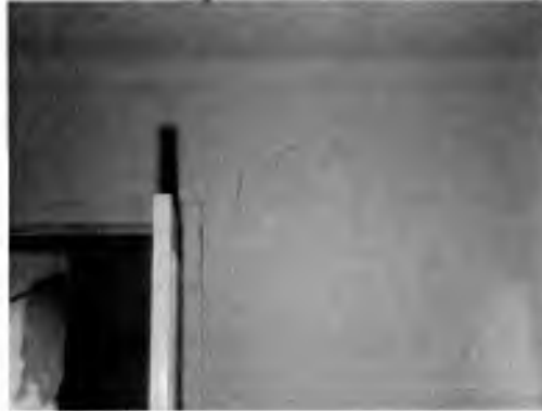
Photo 43: Rear RHS Bedroom Cracking to 2 mm.
