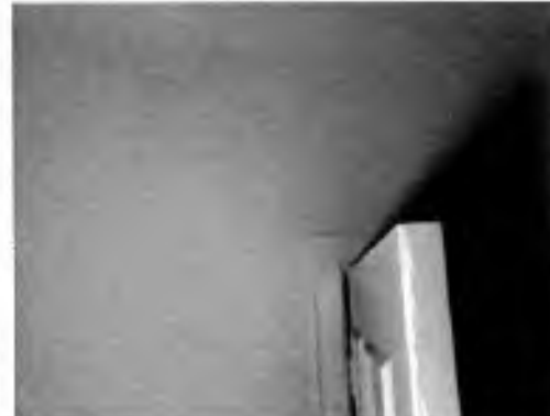
Photo 47: RHS Bedroom 1.0 mm
