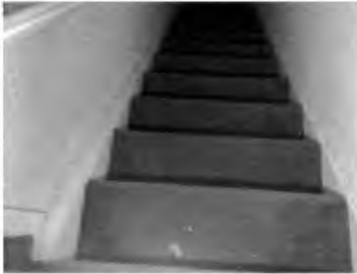
Photo 48: Stair Gap to RHS Filled
