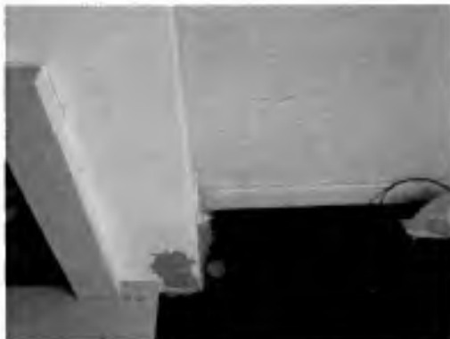
Photo 33: Cracking to 1.0mm in RHS Gable.
