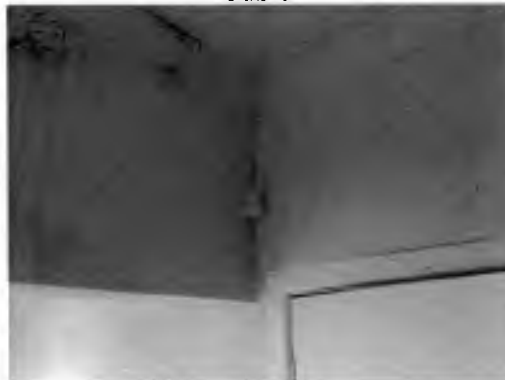
Photo 35: Kitchen Pantry under Stairs 5 mm Crack
