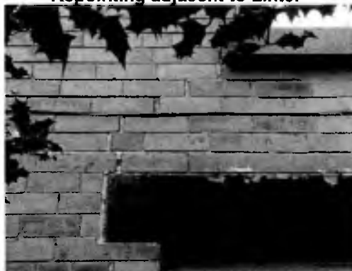
Photo 13: Old Pointing over RHS GF Window
