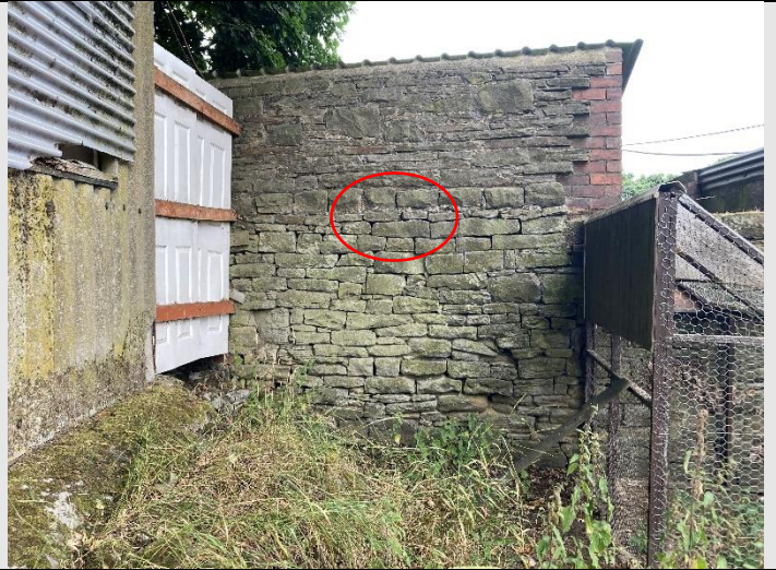
Figure 32. Southern elevation of Building 13 with missing mortar providing gaps in stonework.
