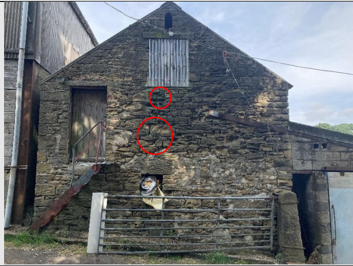
Figure 7. Southern elevation of Building 1 showing two storey stone wall. Gaps in mortar providing roosting potential.
