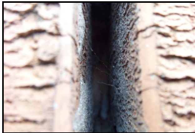
Figure 5. Gaps in external wall of Building B leading to cavity.
