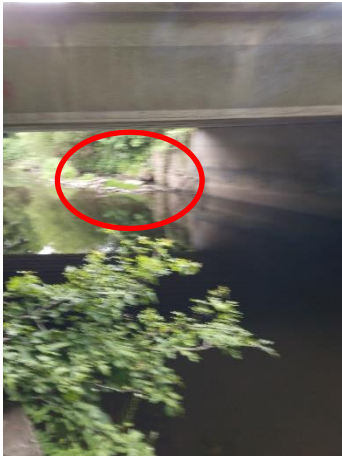
Figure 24: Bridge Smithies Lane (area suitable for holt marked with red keyline)
