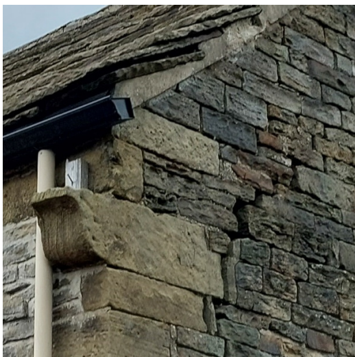
Front elevation cracks to be closed
