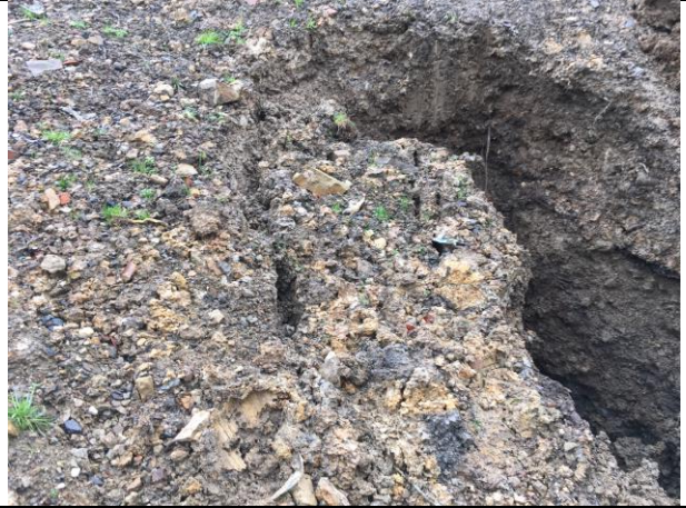
Collapsing excavations within trial pit reference STP04
