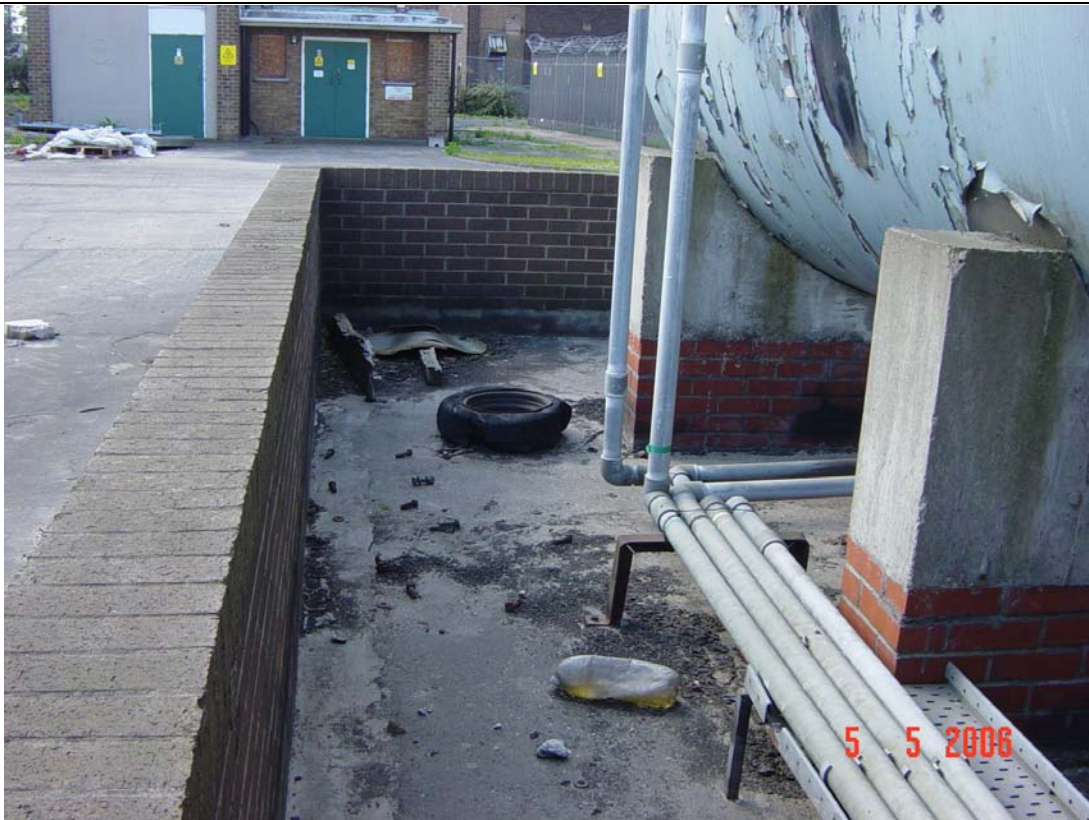
Plate 5 – Redundant tank close up with electricity sub-station in the background.
