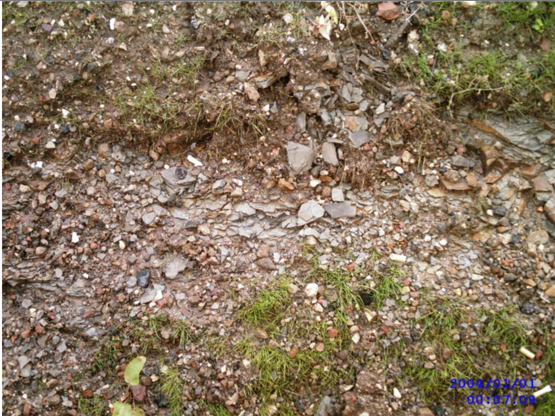
Plate 13 – Fractured bedrock immediately under the slope surface.
