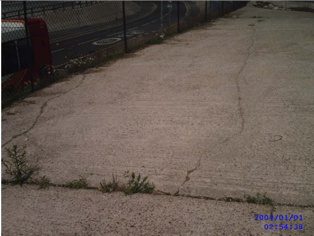
Plate 11 - Fractures in the roadway above the slope.
