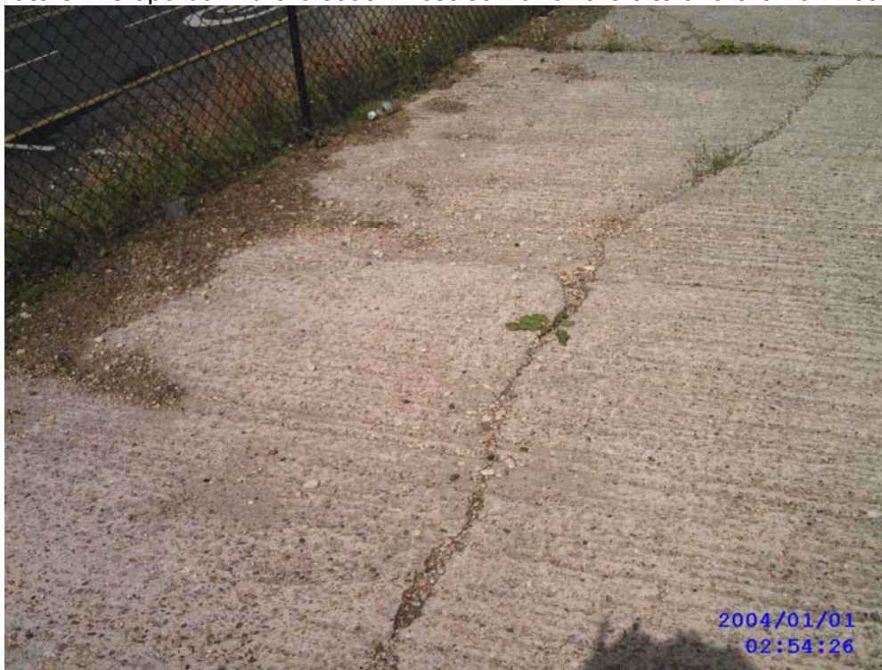
Plate 10 – Fractures in the roadway above the slope.
