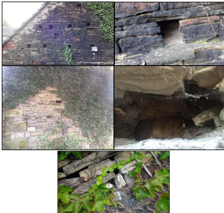
Figure 6. Gaps, cracks and cavities within the walls of the building.
