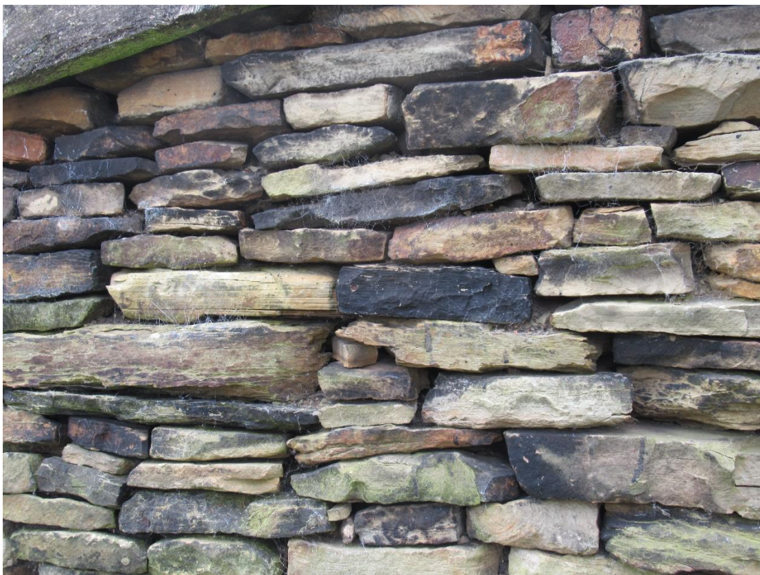
Photograph 6 – Gaps within the drystone walls.
