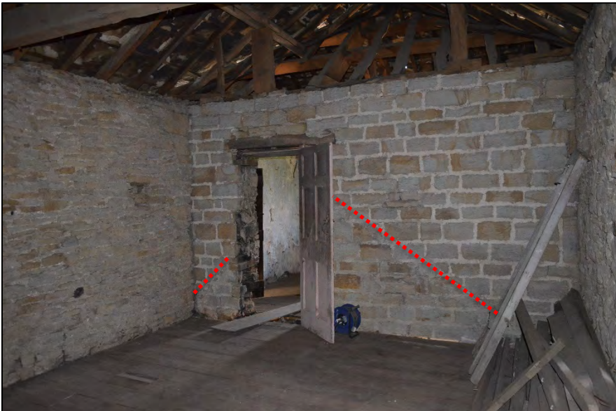
Figure 19: View of first floor room F3 , looking north-west noting roof scar
