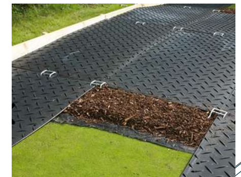
Figure 3: Example of Temporary Ground Protection Boards (GroundGuards) with membrane and woodchip layer:
