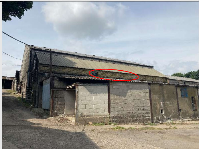
Figure 8. Eastern elevation of Building 1 with gaps in mortar providing roosting potential.
