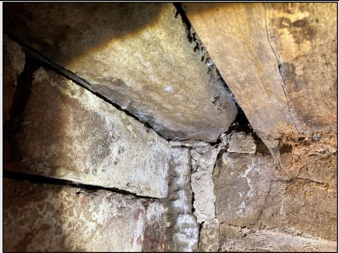
Figure 10. Internal gap in timber lintel with suitability within Building 1.
