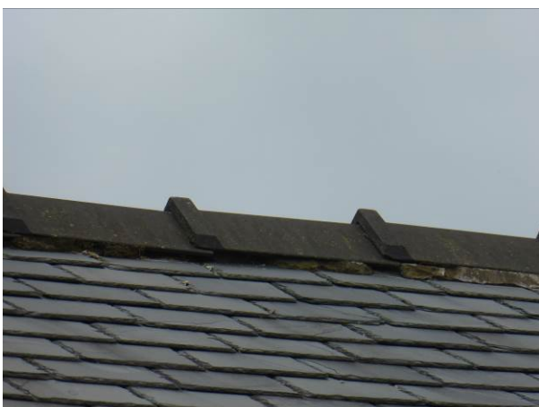
Fig. 17. Old Top Office – gaps beneath ridge tiles.
