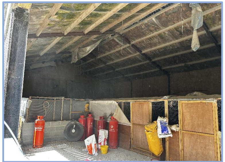
INTERNAL FRAME VIEW
