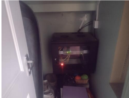
Network Cabinet in understairs cupboard in Spencer Wing
