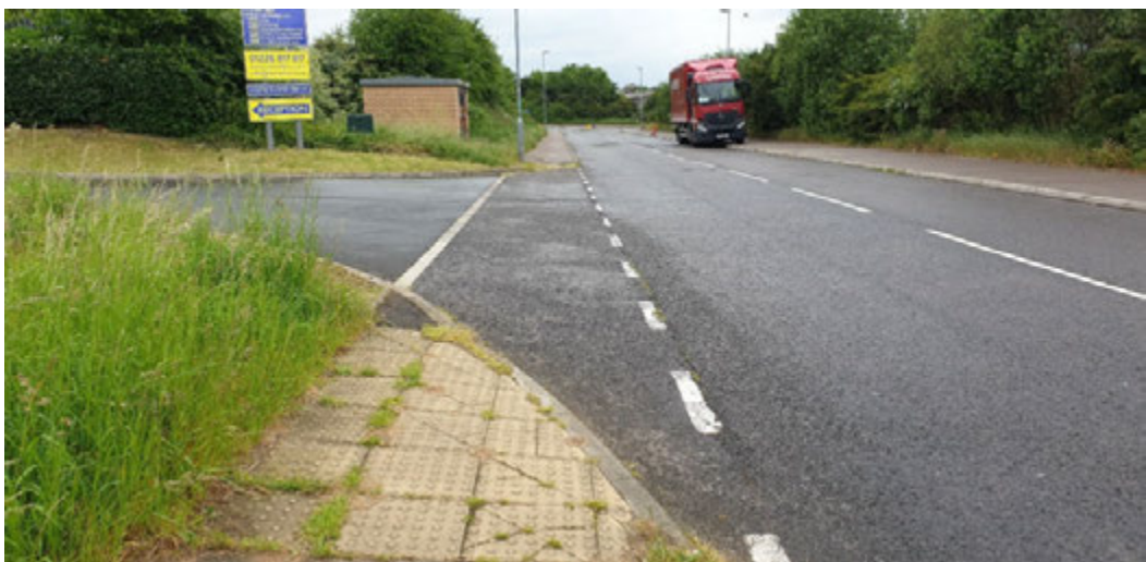
Figure 11 - Western side of entrance. Heavy vegetation in between tactile pavers.
