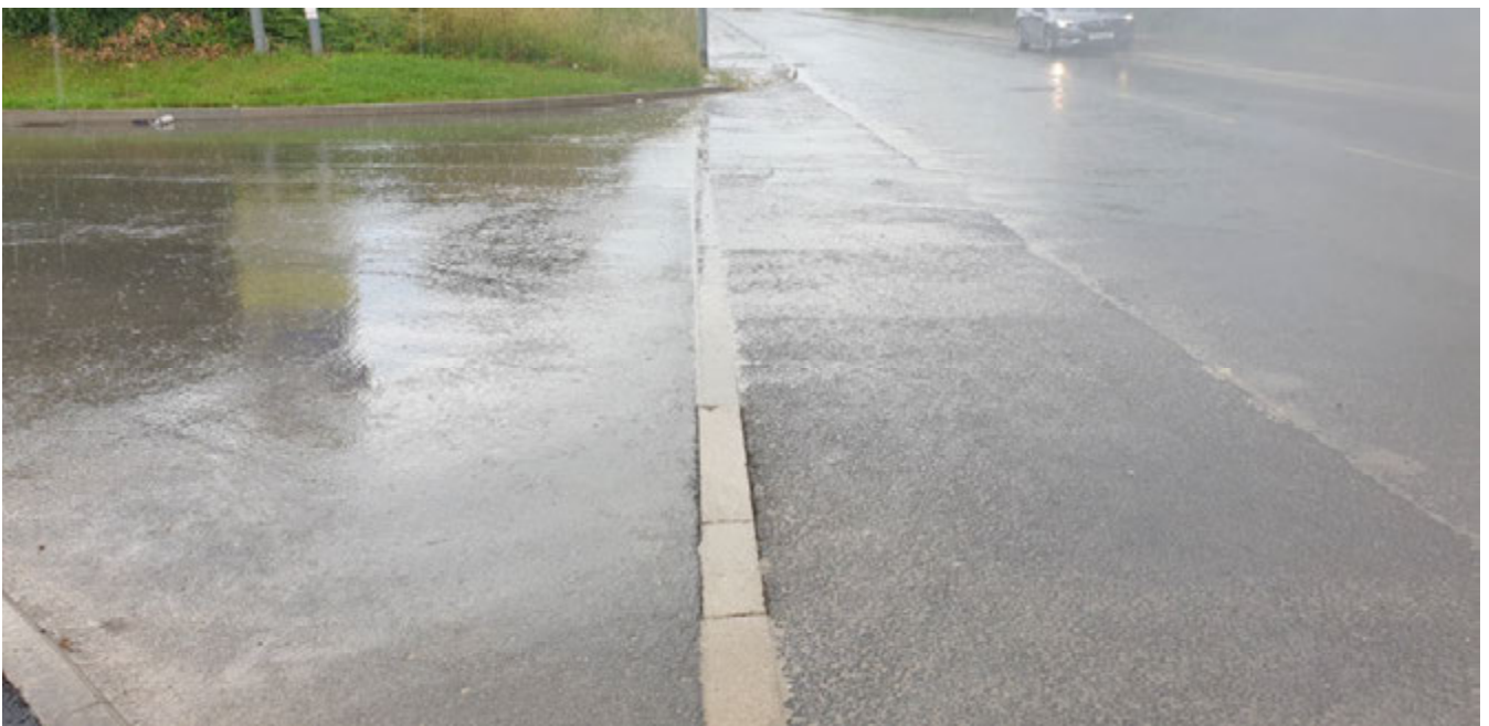
Figure 8 - Loose channel blocks at back of access to Plot 4B - this will need replacing. Identified pre-works refer to Figure 12 Appendix B.
