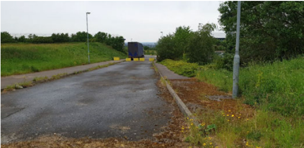
Figure 47 - Footway on eastern side heavily covered in moss.
