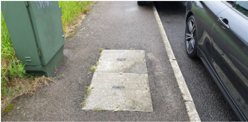
Figure 9 - BT chamber in southern footway.
