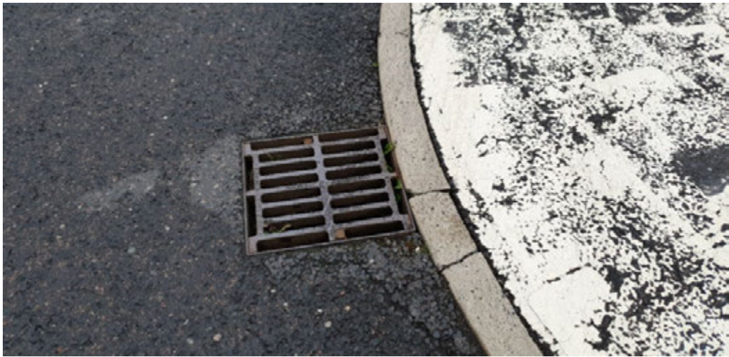
Figure 21 - Loose kerbing adjacent gully on island.
