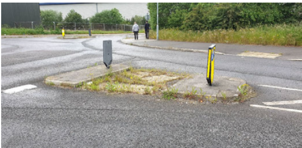
Figure 17 - View across pedestrian crossing point on eastern leg of mini roundabout. Very heavy vegetation on tactile paving in island.
