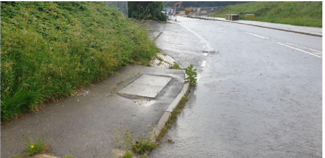
Figure 24 - Footway surrounding BT cover is sunken, this was present prior to works commencing and shown in the pre-start inspection photos. Refer to Figure 27 appendix B.
