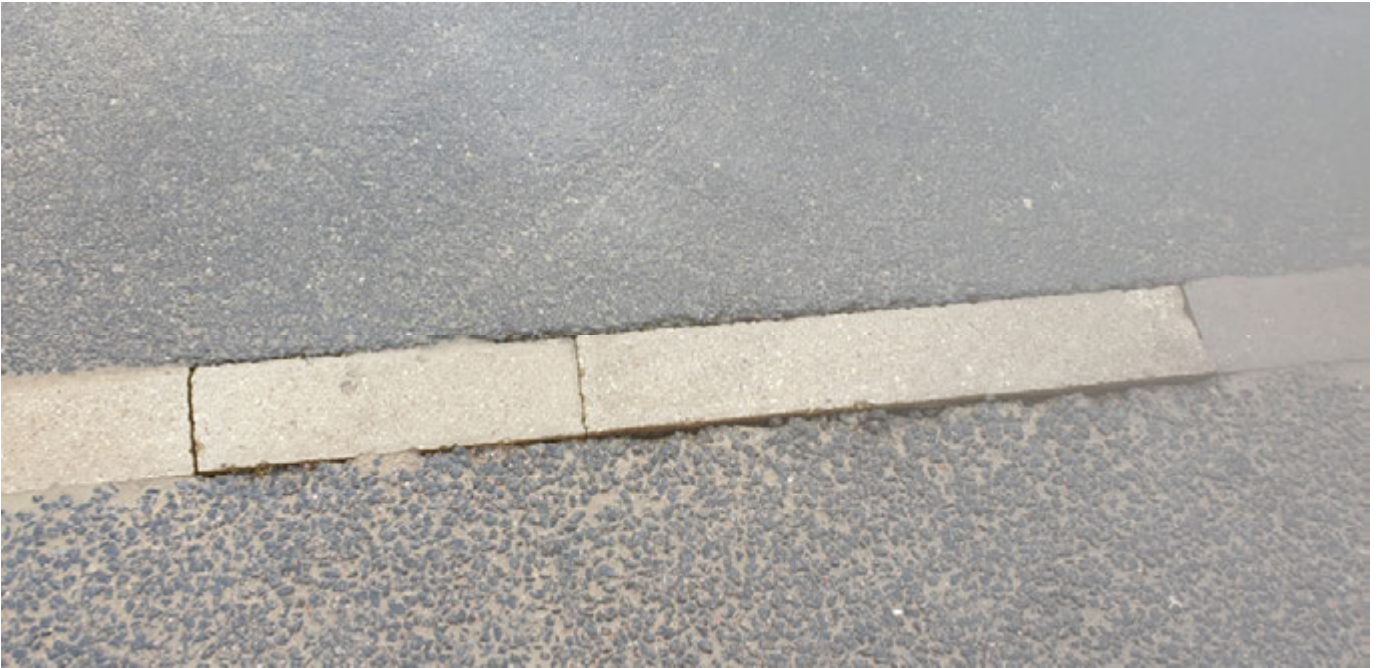
Figure 9 - Close up of damaged channel blocks. Identified pre-works refer to Figure 12 Appendix B.
