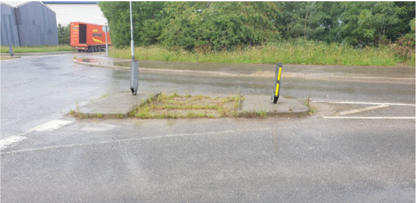
Figure 13 - Mini roundabout island on eastern approach.
