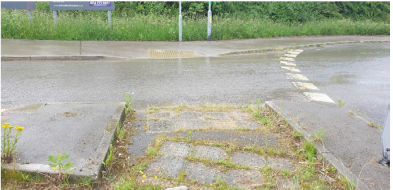
Figure 22 - View across island on southern leg of roundabout. Paving overgrown with weeds and vegetation.
