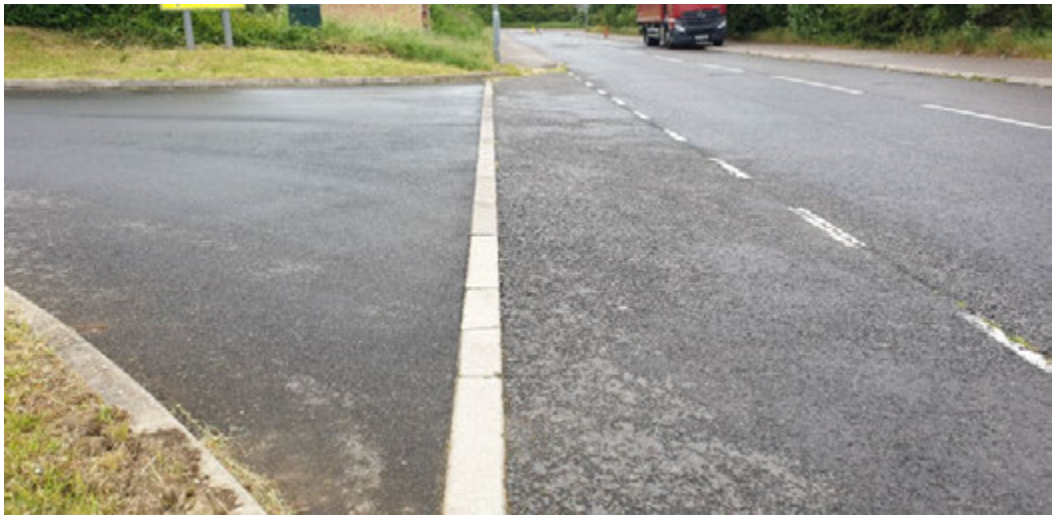
Figure 12 - Existing demarcation channels at rear of Highway boundary. Some channel blocks are loose and rocking.
