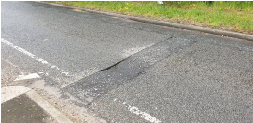
Figure 239 - Failed reinstatement on Ryecroft Bank to the north of junction with Ashroyds Way.
