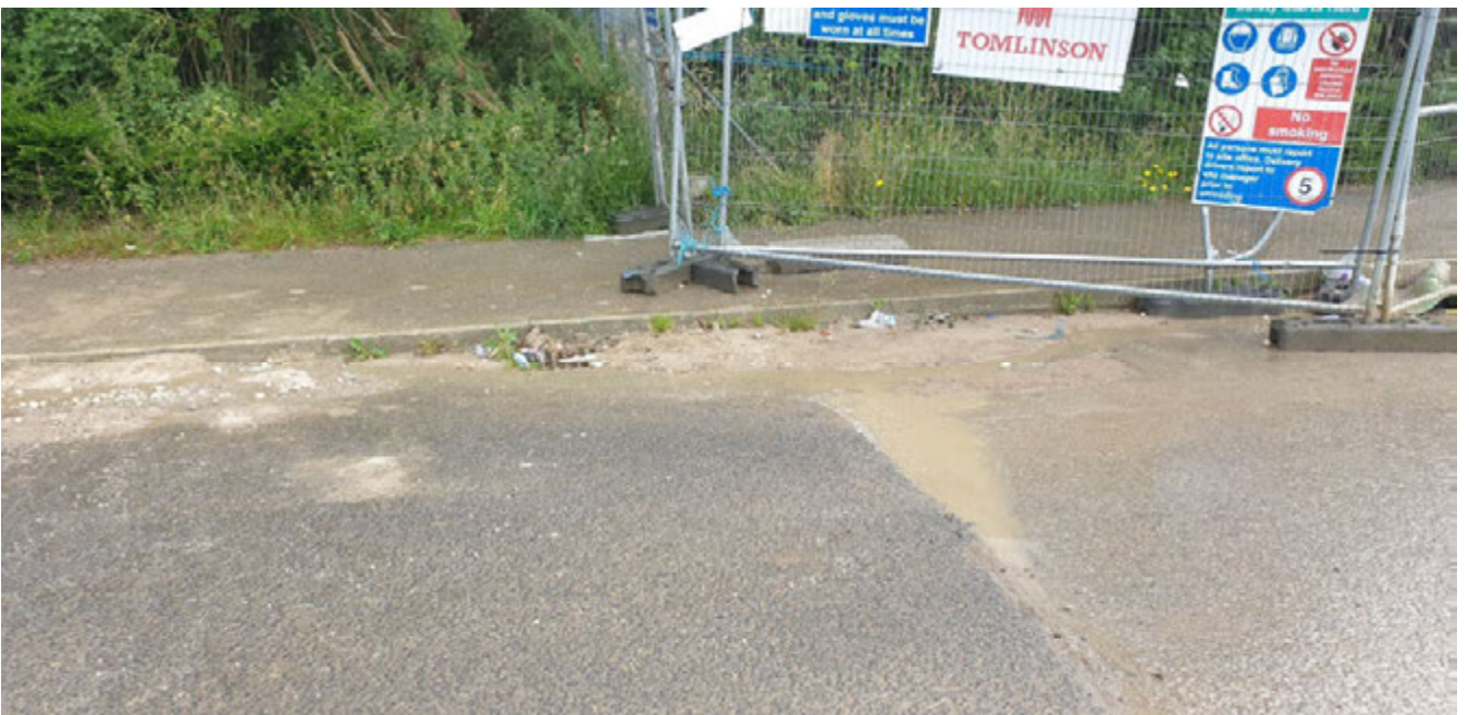
Figure 28 - Debris in channel adjacent gully. Note this is within the S38 agreement area.
