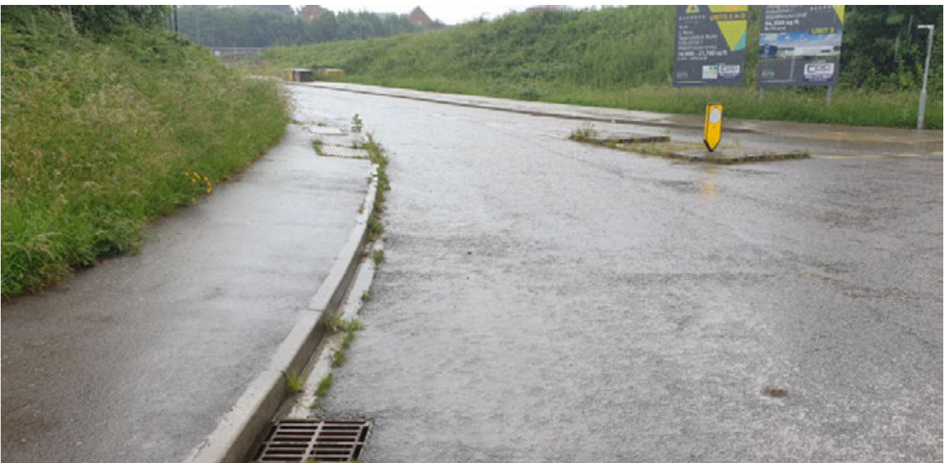
Figure 14 - View to southern leg from roundabout to Plot 5. Note missing bollard, this was missing prior to the works starting. Refer to Figure 25 Appendix B
