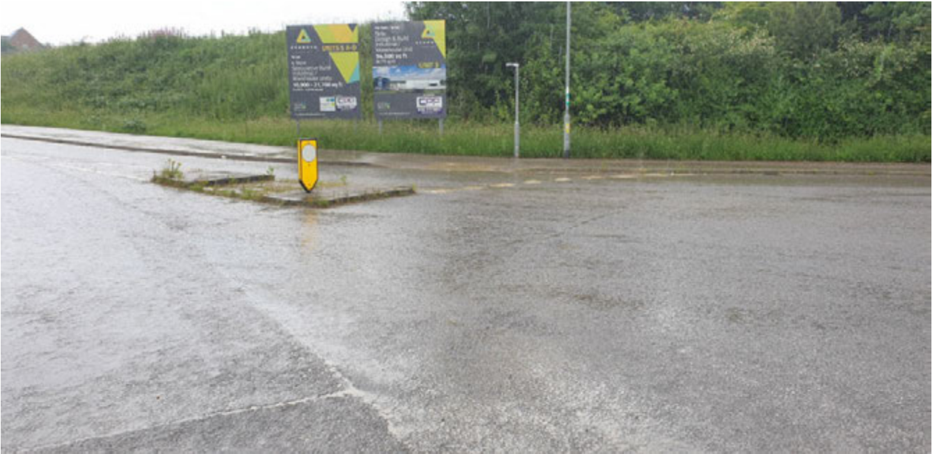
Figure 15 - View to southern leg from roundabout to Plot 5. Note missing bollard, this was missing prior to the works starting. Refer to Figure 25 Appendix B
