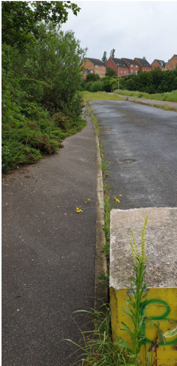
Figure 44 - Eastern channel looking south from concrete blocks. Vegetation encroaching over footway.
