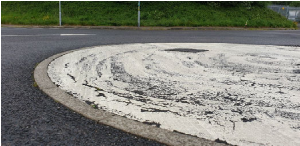
Figure 33 - Depression in mini-roundabout surfacing.
