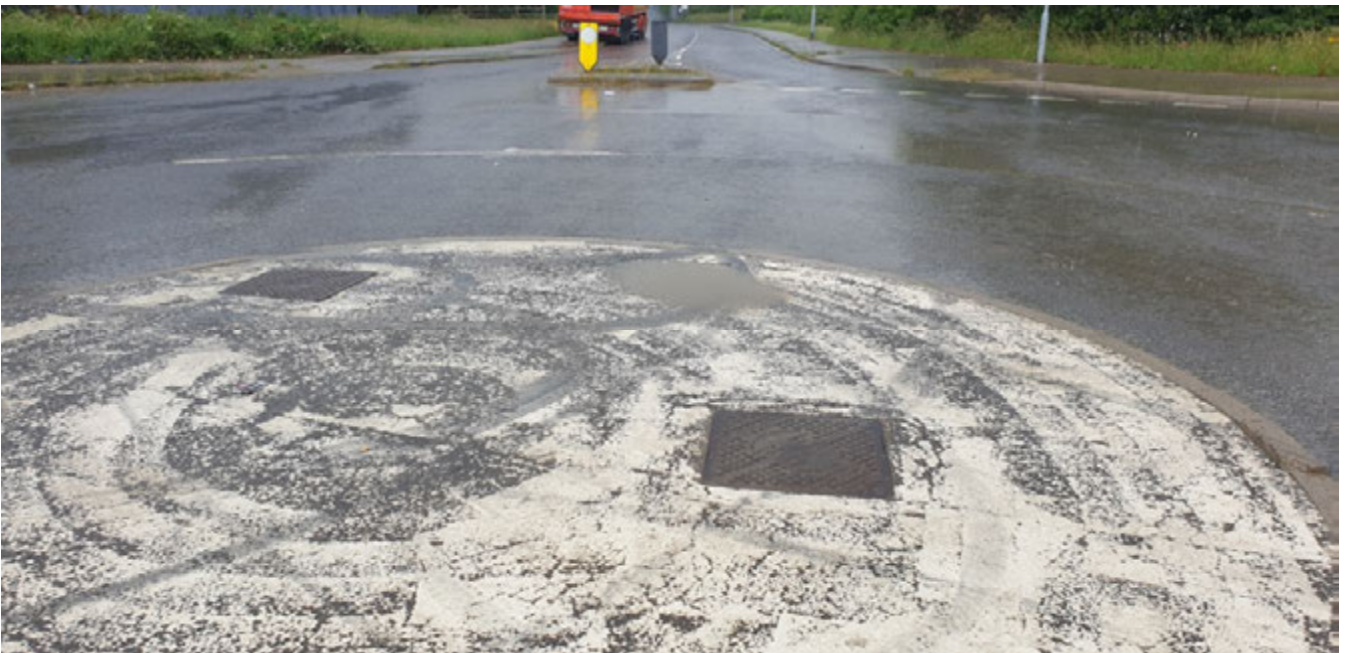
Figure 20 - View of centre island at roundabout. Note the depression was present prior to works starting at was noted on the pre-start report. Refer to Figures 21,32,33 – Appendix B.
