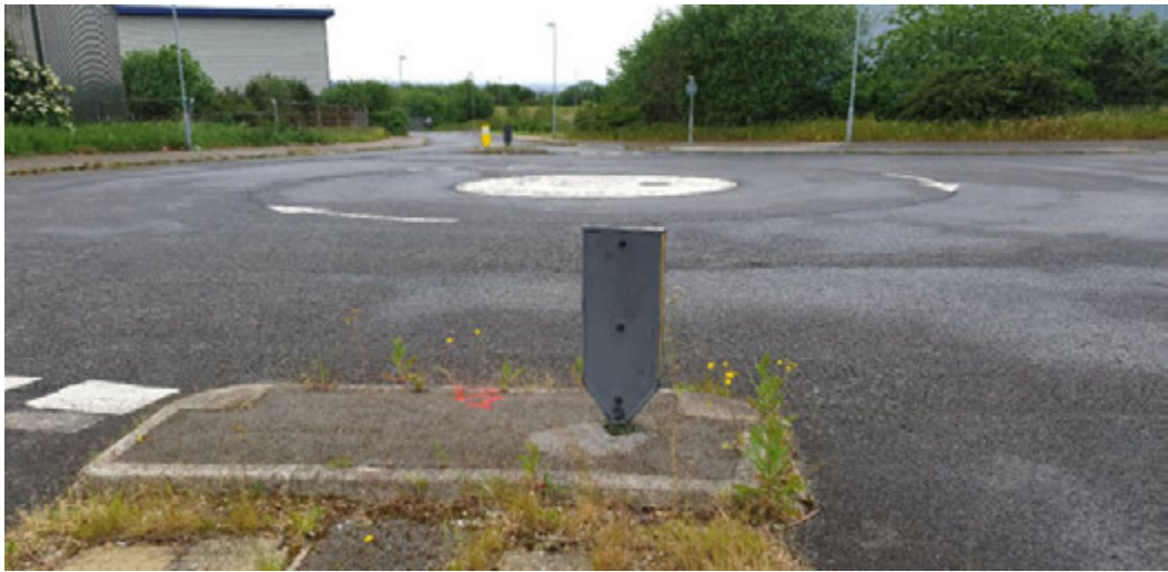
Figure 24 - View from pedestrian island on southern leg. Heavy vegetation in kerb lines/tactile pavers.
