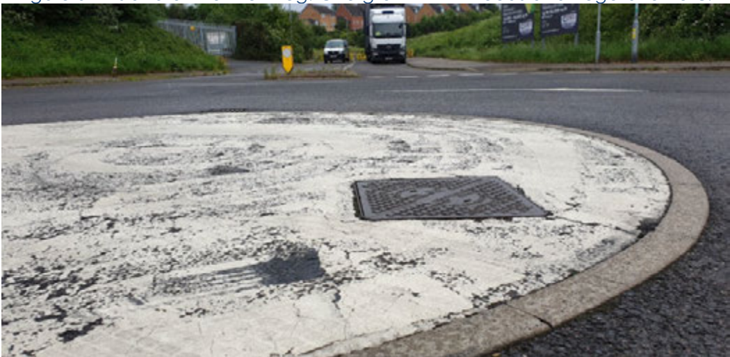
Figure 32 - Depression in mini-roundabout island from vehicle overrun into the northern leg. Slight breaking up of surfacing around manhole cover.
