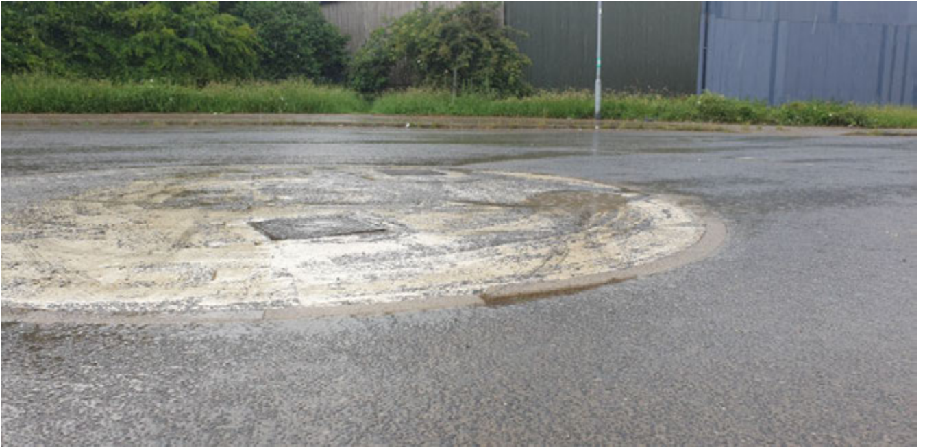
Figure 17 - View of centre island at roundabout. Note the damaged kerbs were present prior to works starting at was noted on the pre-start report. Refer to Figures 21,32,33 – Appendix B.
