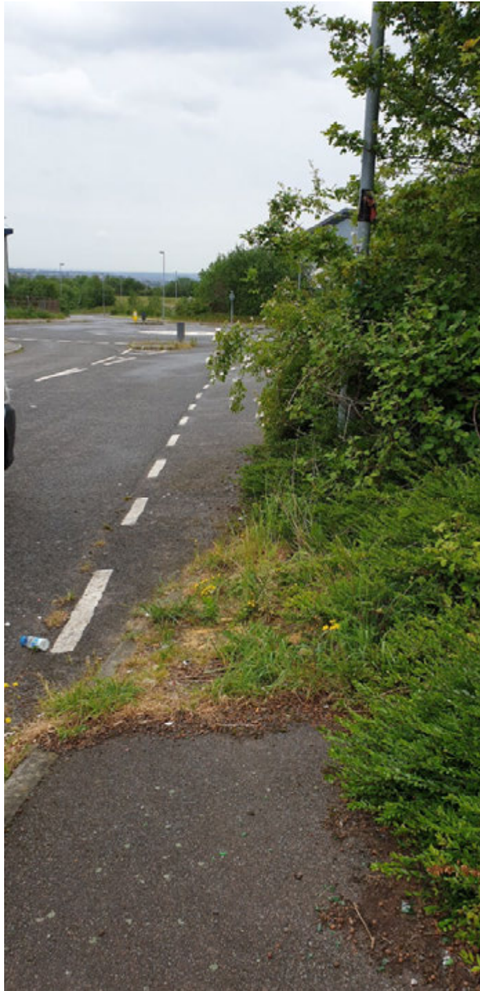
Figure 45 - Tactile crossing across access. Vegetation encroaching.
