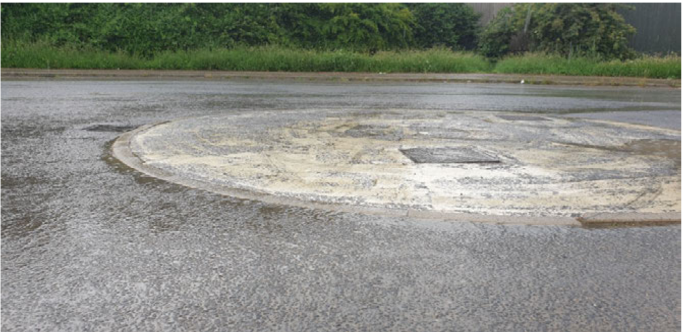
Figure 18 - View of centre island at roundabout. Note the damaged kerbs were present prior to works starting at was noted on the pre-start report. Refer to Figures 21,32,33 – Appendix B.
