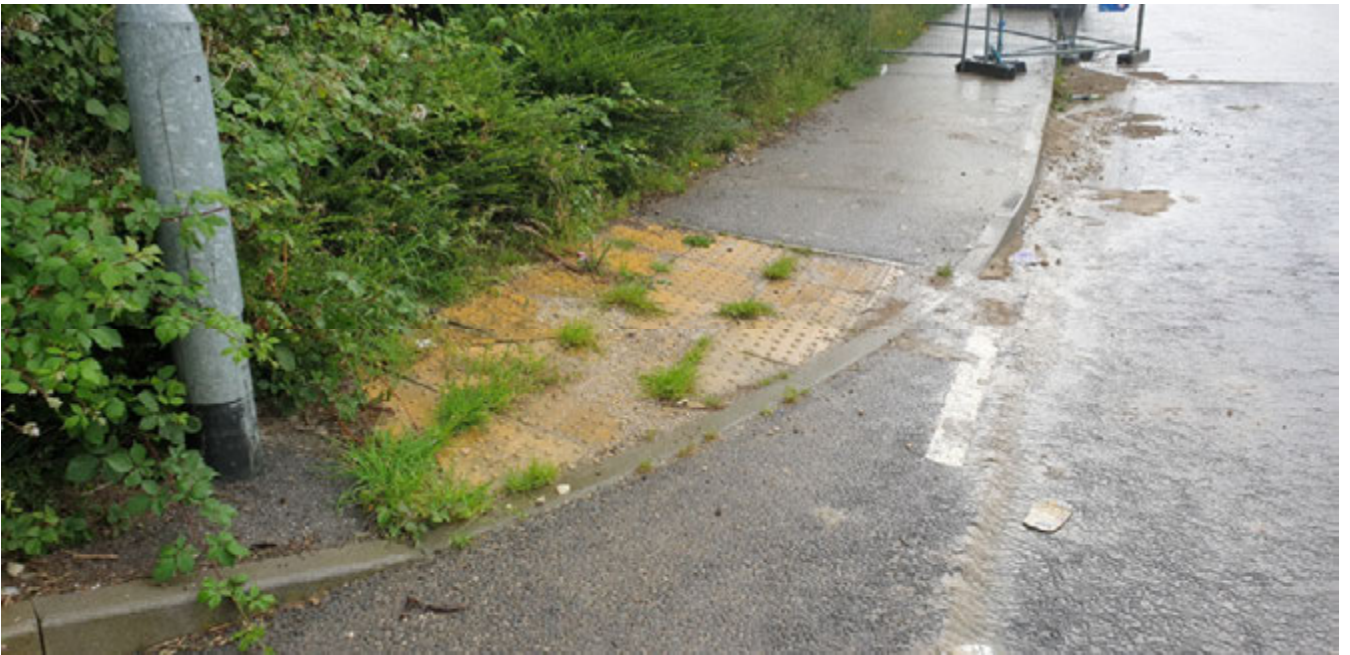
Figure 25 - View of tactile pavers to north of Storefirst entrance. Some vegetation has been removed. Tactile pavers are uneven, note these are located in the are to be adopted under S38 agreement. Refer to Figure 45 Appendix B.
