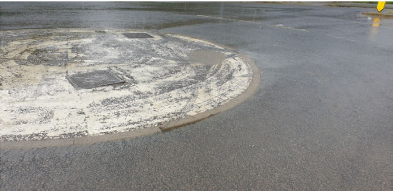
Figure 16 - View of centre island at roundabout. Note the damaged kerbs were present prior to works starting at was noted on the pre-start report. Refer to Figures 21,32,33 – Appendix B.
