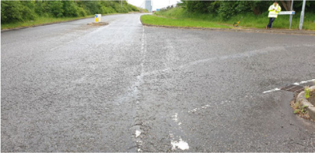
Figure 40 - View north of westbound lane into Ashroyds Way. Some minor chipping loss in the surface course. All junction lining is worn out.
