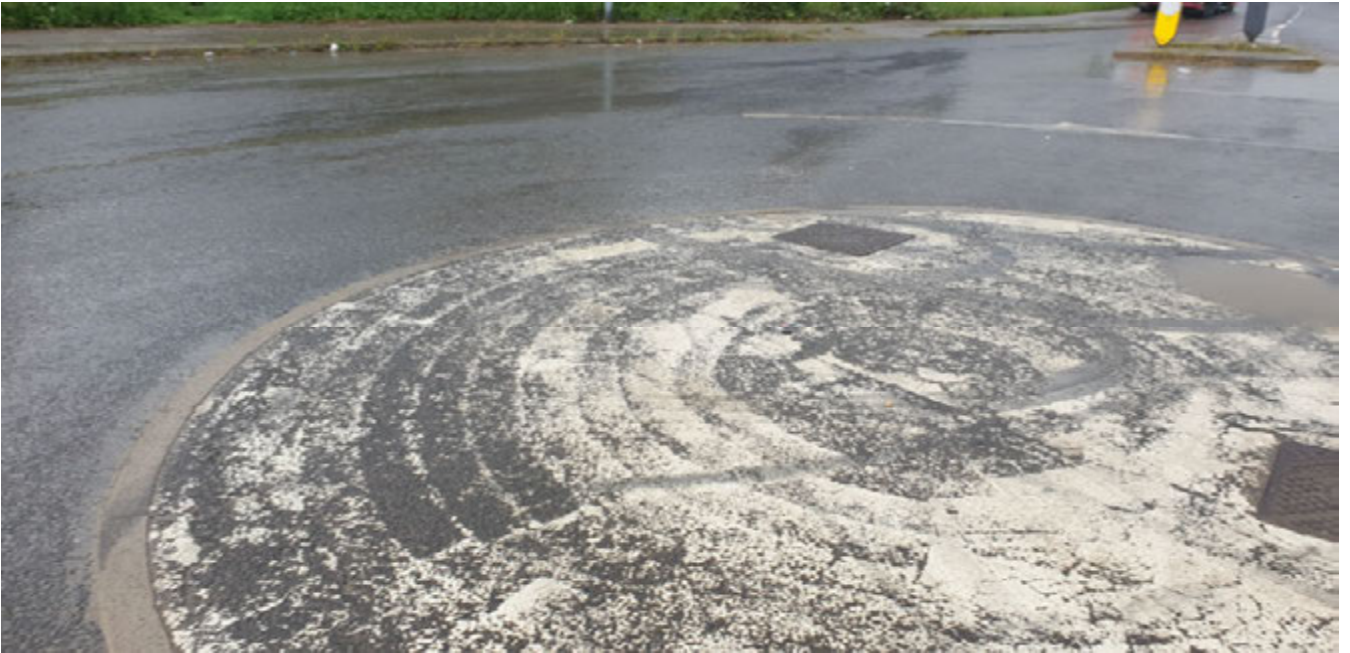
Figure 19 - View of centre island at roundabout. Note the depression was present prior to works starting at was noted on the pre-start report. Refer to Figures 21,32,33 – Appendix B.
