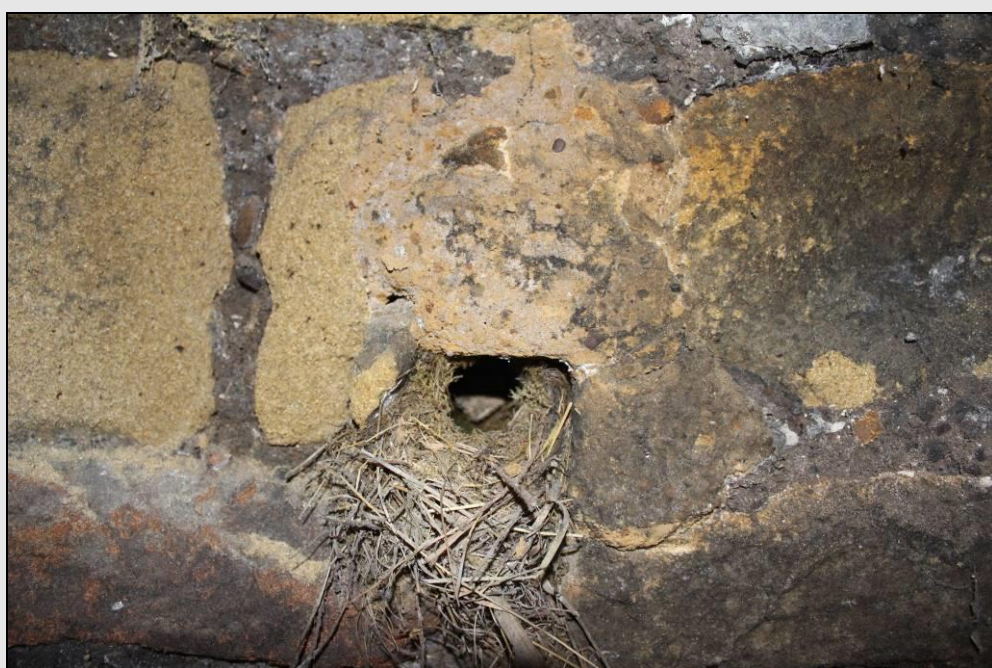
Figure 21. Internal view of hole in south-east wall of Building 2, showing disused nest.
