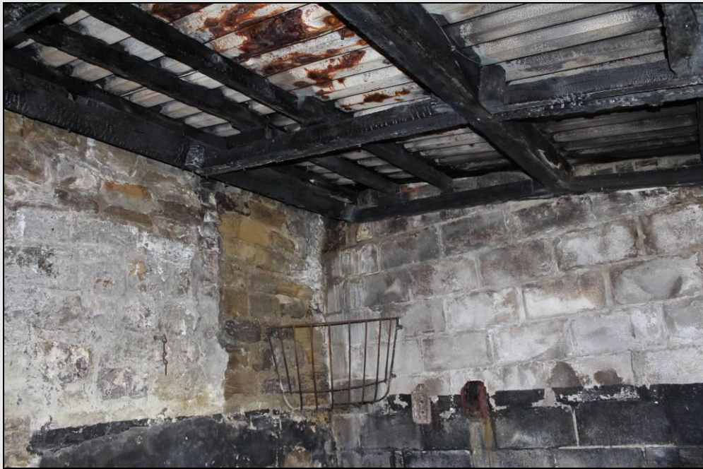
Figure 38. Internal view of northern end of Building 4A, showing fire damage to walls and roof.
