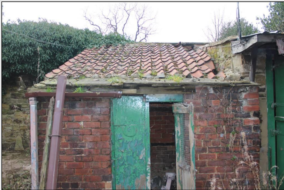
Figure 39. External view of north-east roof elevation of Building 4B, showing missing and lifted roof tiles.
