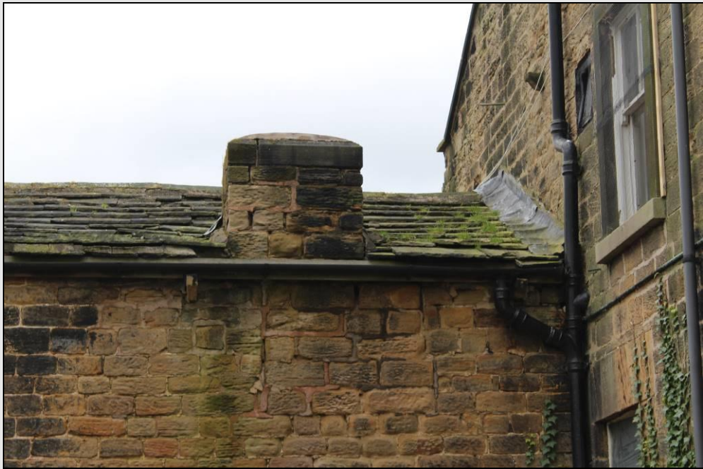
Figure 14. External view of south-western roof elevation of Building 1B, showing missing, slipped and lifted tiles.
