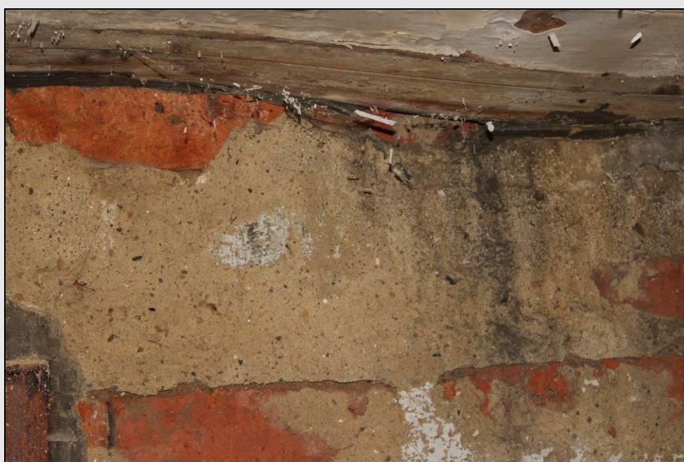
Figure 16. Internal view of loft space in Building 1B, showing gaps between sarking and internal wall, providing potential entrance point between loft space and void between roof tiles and sarking.
