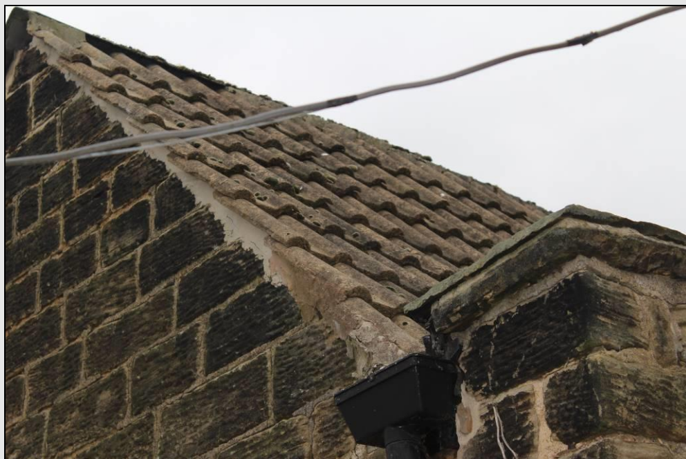
Figure 28. External view of the south-east roof elevation of Building 3B, showing gaps in mortar below ridge tiles.
