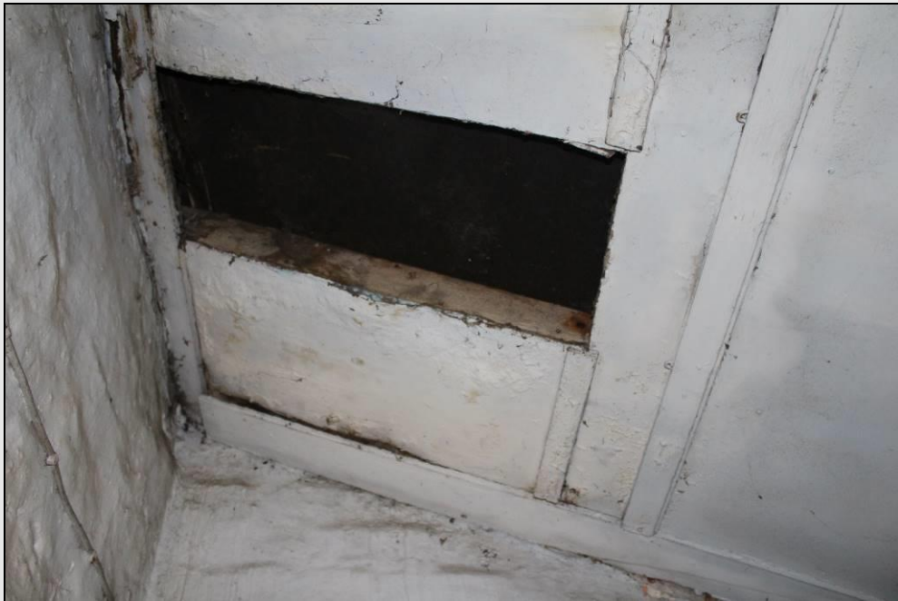
Figure 40. Internal view of Building 4B, showing missing wooden panels which reveal the underlining of the roof tiles.
