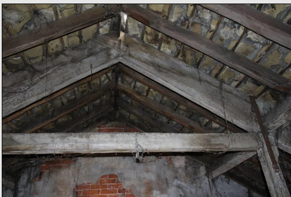
Figure 10. View of loft space within Building 1A, showing potential entry point in roof apex under lifted/missing tile.
