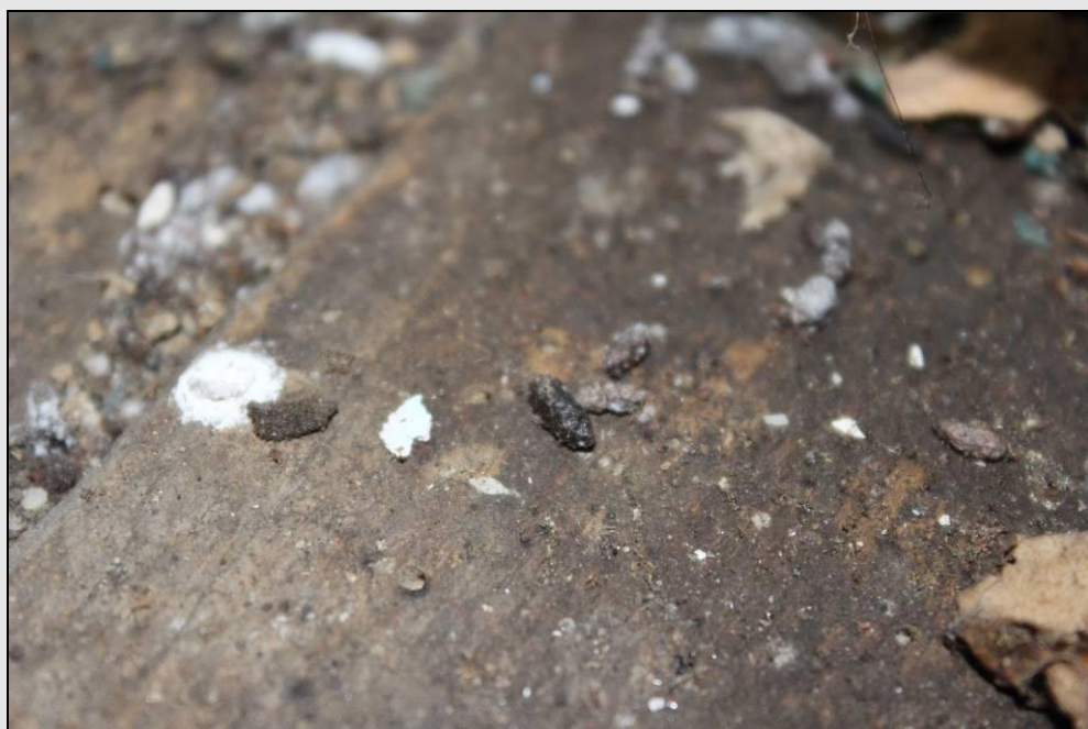
Figure 31. Internal view of the ground floor of Building 3B, showing a potential bat dropping.
