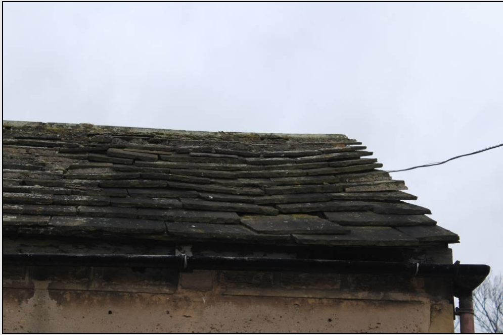
Figure 24. External view of south-east roof elevation of Building 3A, showing slipped and lifted tiles.
