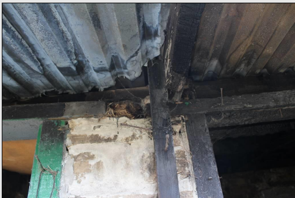
Figure 37. External view of north-east face of Building 4A, showing disused bird's nest between two beams.
