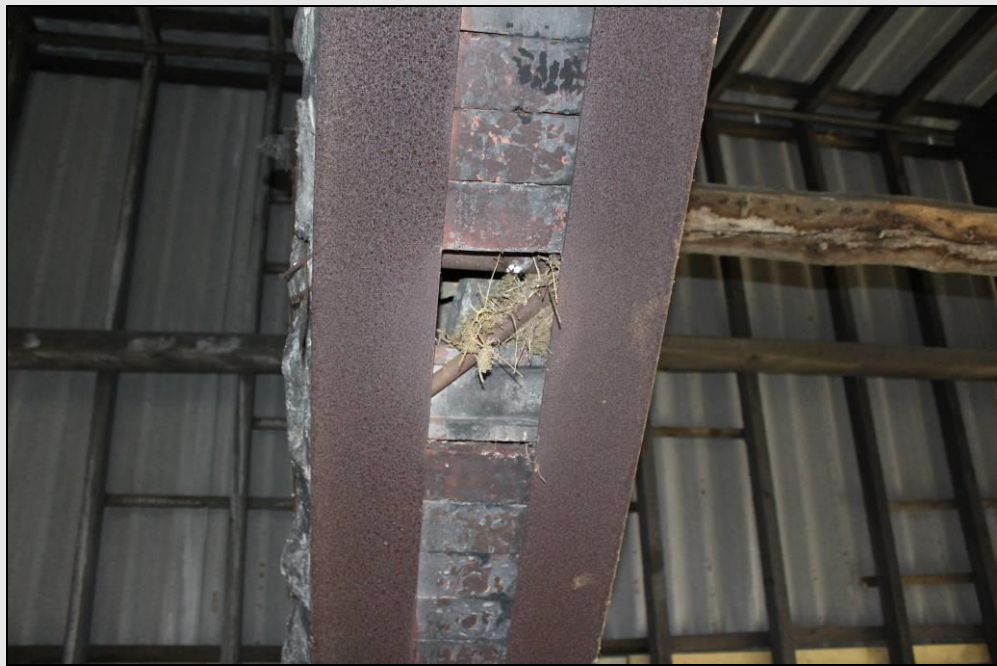
Figure 22. View of gap in one of the internal roof beams of Building 2, showing potential nesting materials.
