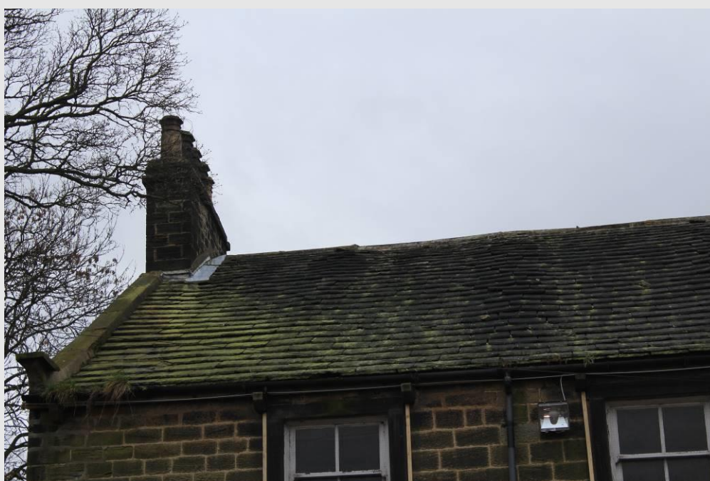
Figure 8. External view of the north-eastern roof elevation, showing lifted tiles.
