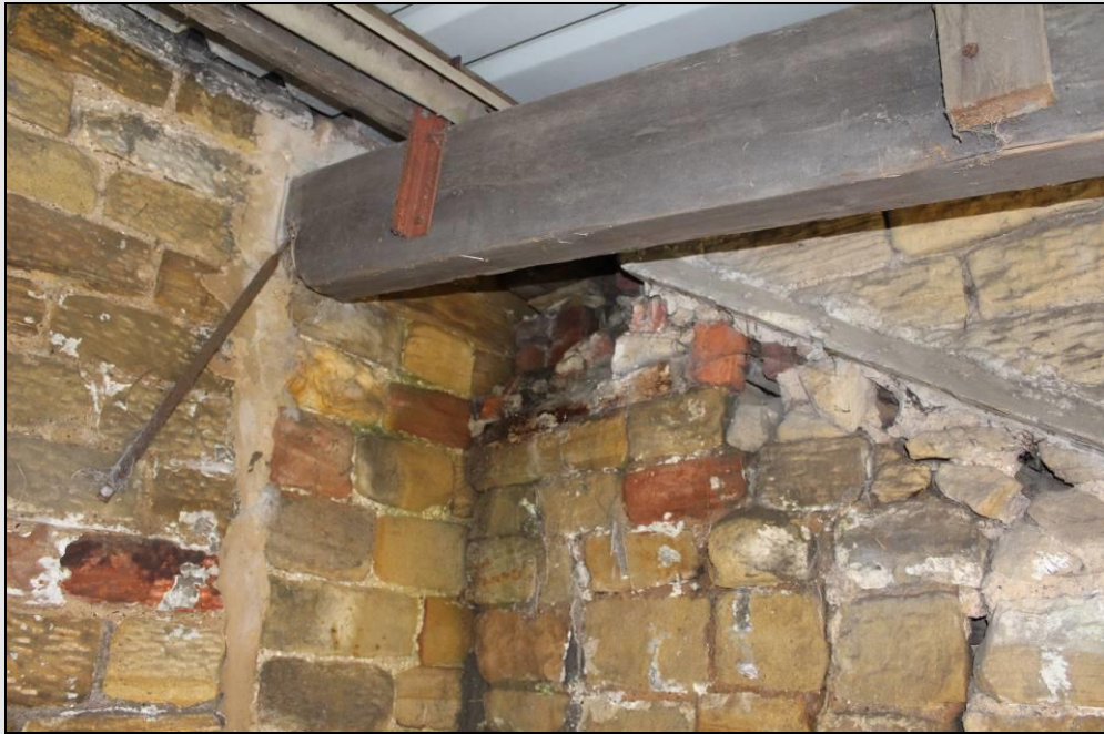
Figure 34. Internal view of south-west wall of Building 3C which attached to Building 3B, showing large area of missing stone and mortar leading to cavity of wall.
