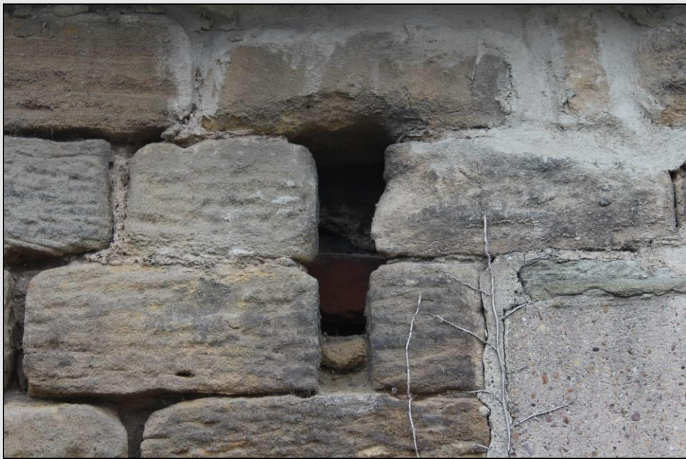
Figure 18. External view of south-east face of Building 2, showing a hole leading to the wall's cavity.
