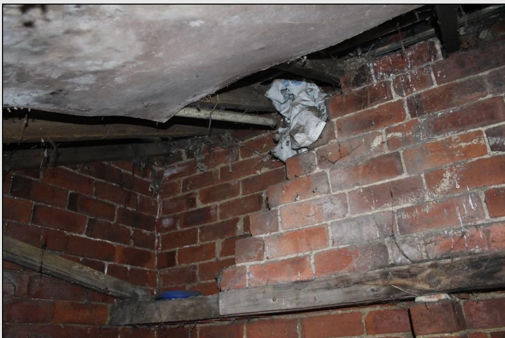
Figure 41. Internal view of Building 4B, showing wooden boarding of roof falling down and potential gaps between wooden boarding, beams and roof tiles.
