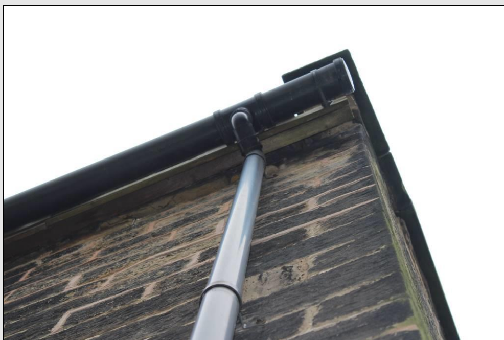
Figure 9. Gap between fascia board and brick wall of Building 1A.
