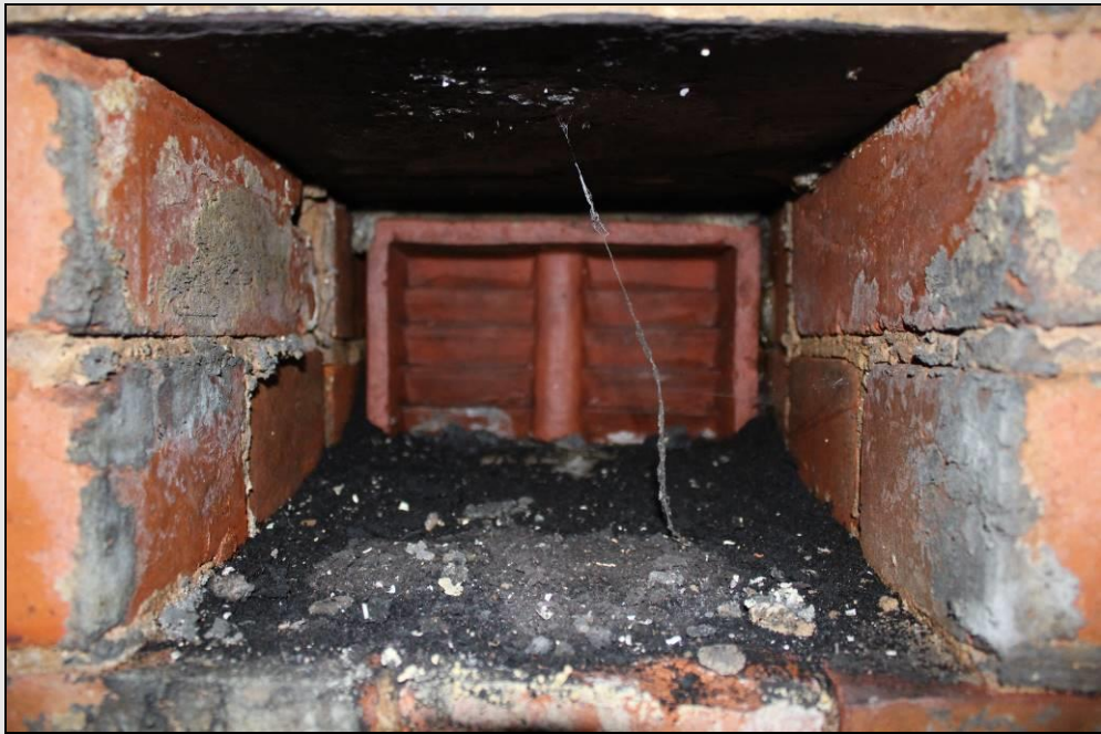
Figure 44. Example of air vent inside Building 5.
