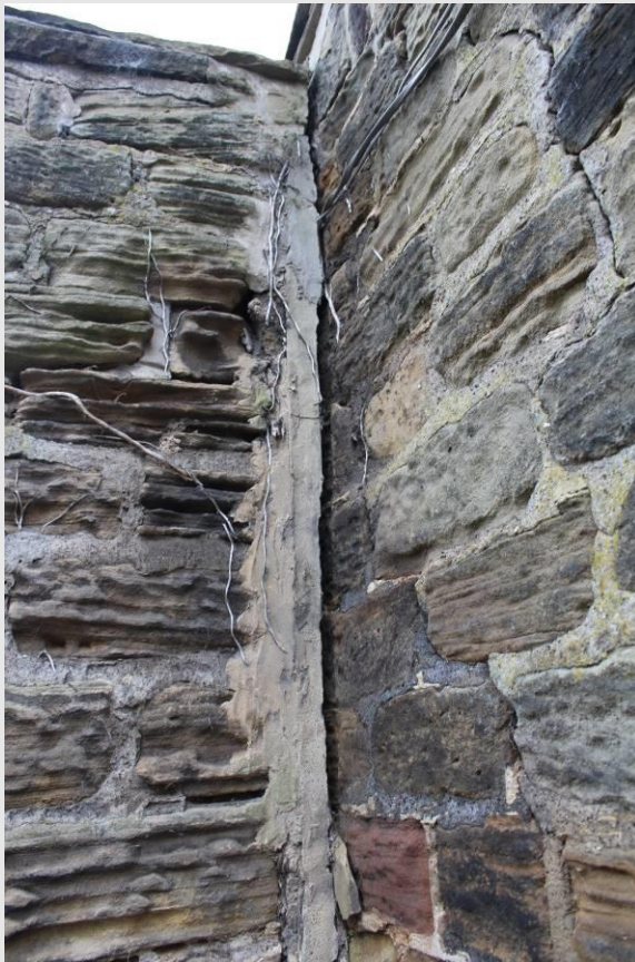
Figure 26. External view of the large crevice between Buildings 3A and 3B.
