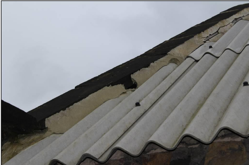
Figure 19. External view of Building 2, showing missing mortar from tiles at gable end of building.
