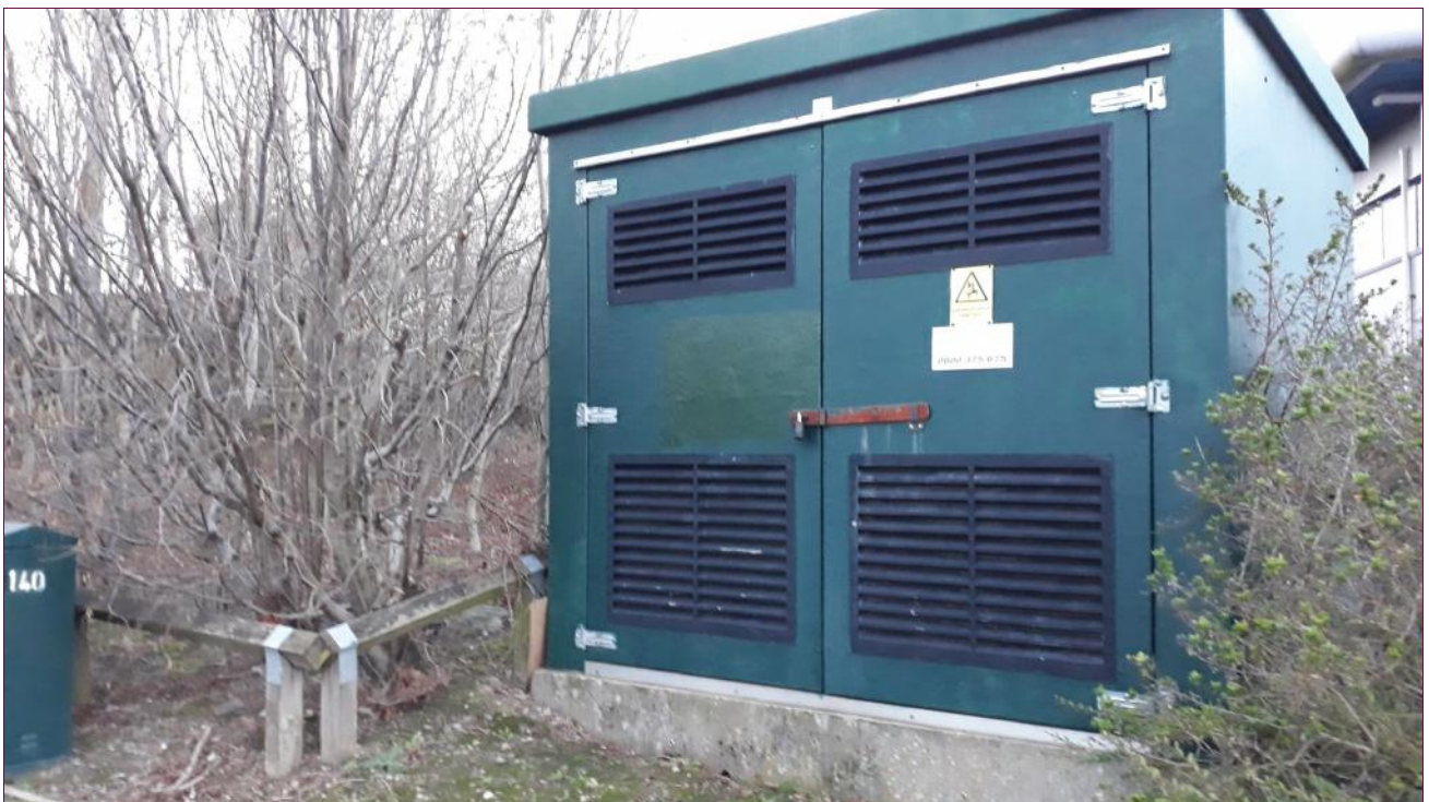
Photograph 8: A substation situated adjacent to the southern corner of the site.
