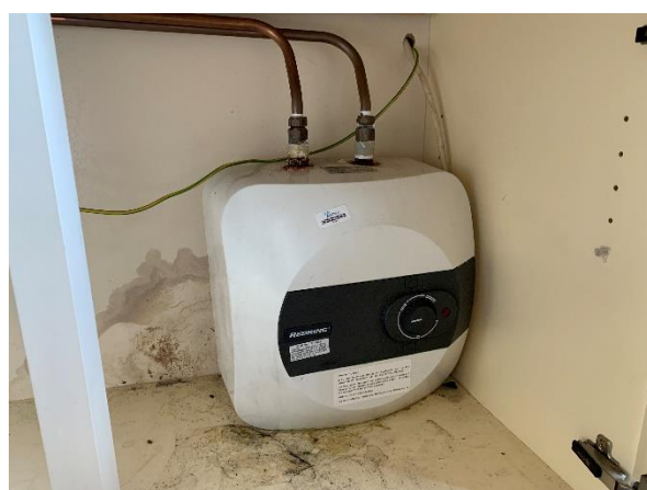
Image 16 Under sink water heater
