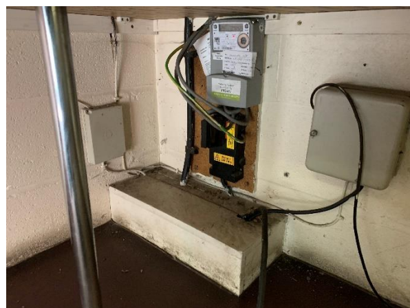
Image 22 Incoming Electricity Supply
