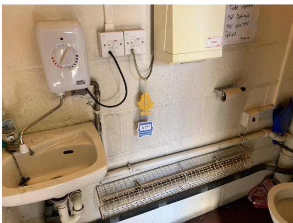
Image 21 Sanitary appliances – water heater
