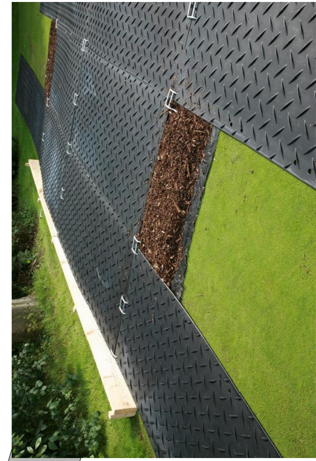
Figure 1. Ground protection will be constructed using no-dig construction principles. This will involve cutting back any understorey vegetation and installing interlinked ground protection boards placed on top of a compression-resistant layer (e.g. 150 mm depth of wood chip), laid onto a geotextile membrane with 300mm overlaps.
