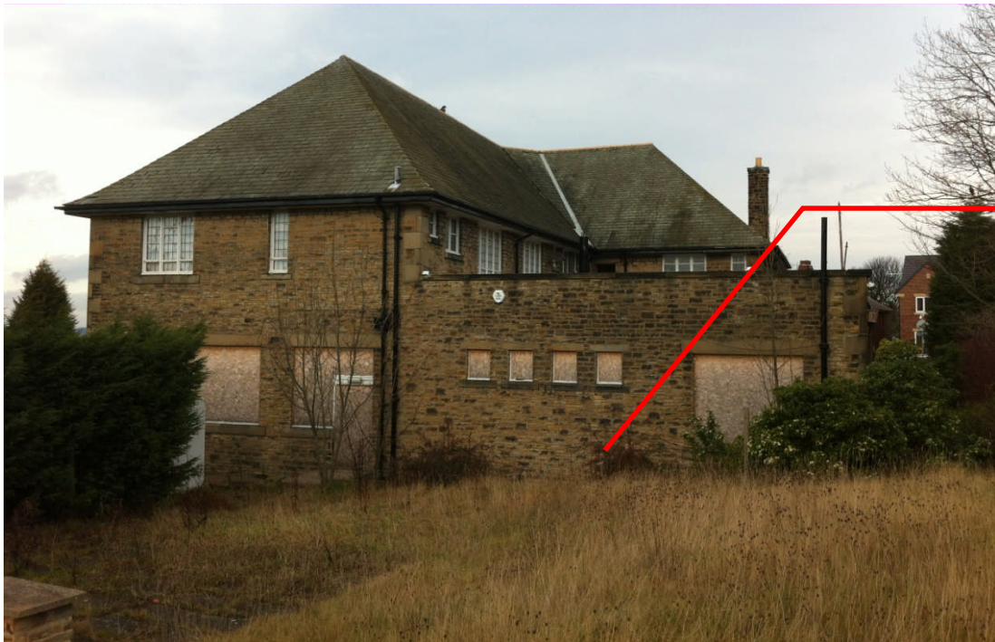
Photo 2.1: The plant location on the rear of the building
