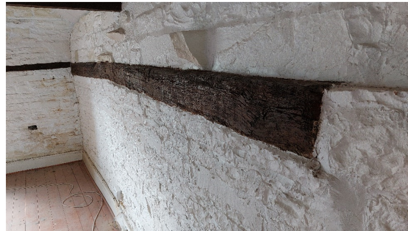
The original stone wall plate is visible in parts where the roof was raised.
