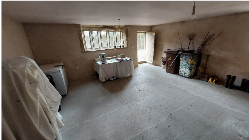
Ground floor room south side, there is a sand cement render to all walls and plasterboard to the ceiling and sand cement screed to the floors
