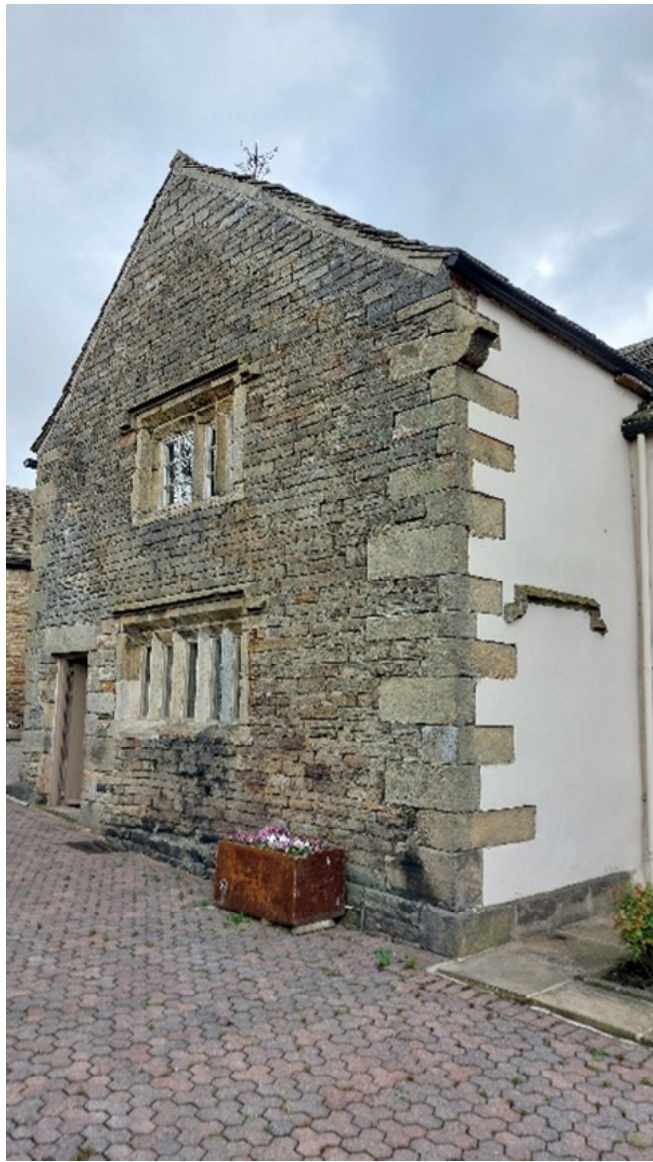
The west wing front (south) elevation, the roof has been raised at some point in its history by approximately 500mm as can be seen from the Kneelers and slight change in stone to the gable
