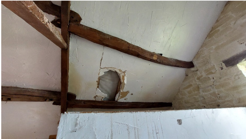
The roof has been renewed at some point with new felt and some insulation and plasterboard finish
