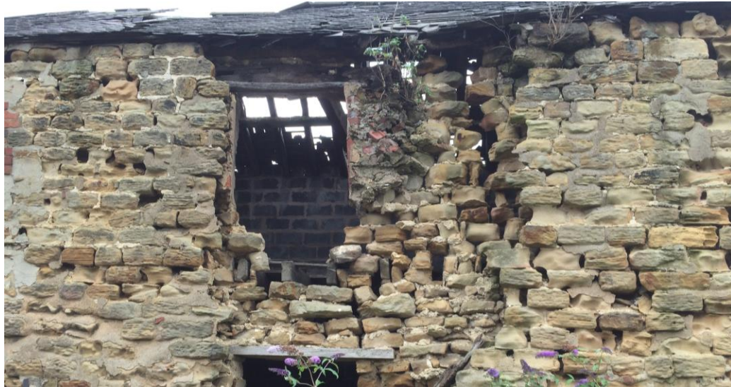
Plate 4 Very dangerous section of west elevation
