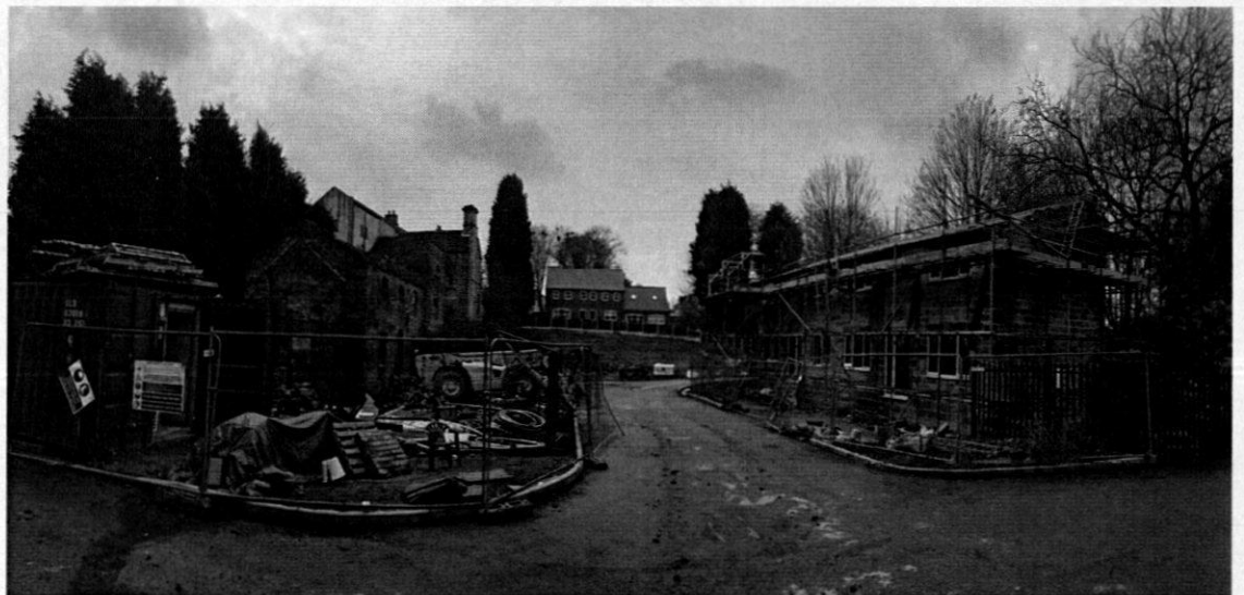
Photograph taken April 2016 showing the construction work approved under application 2006/1116 Thurnscoe Hall is just visible between the two conifer trees left hand side of the photograph.
