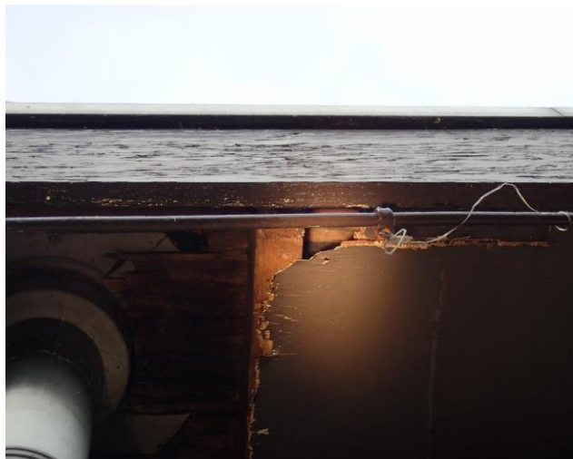
Figure 5 Missing ply under the wooden soffit box of Ward 2
