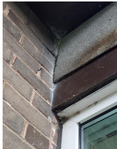
Figure 6 Narrow crack providing entry behind felt on Ward 2 annex
