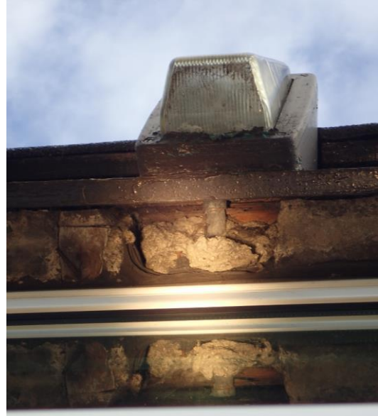
Figure 8 Cracks in brickwork under security light above door
