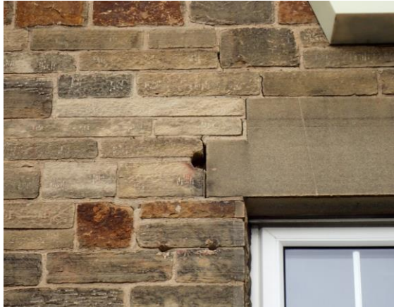
Figure 13 Hole at first floor lintel
