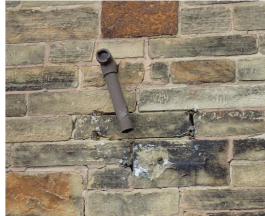
Figure 14 Crack near side entrance
