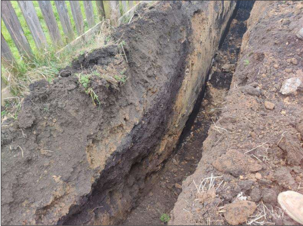
Photo 3: TP01 – Dark coloured infill material within the natural light brown strata.
