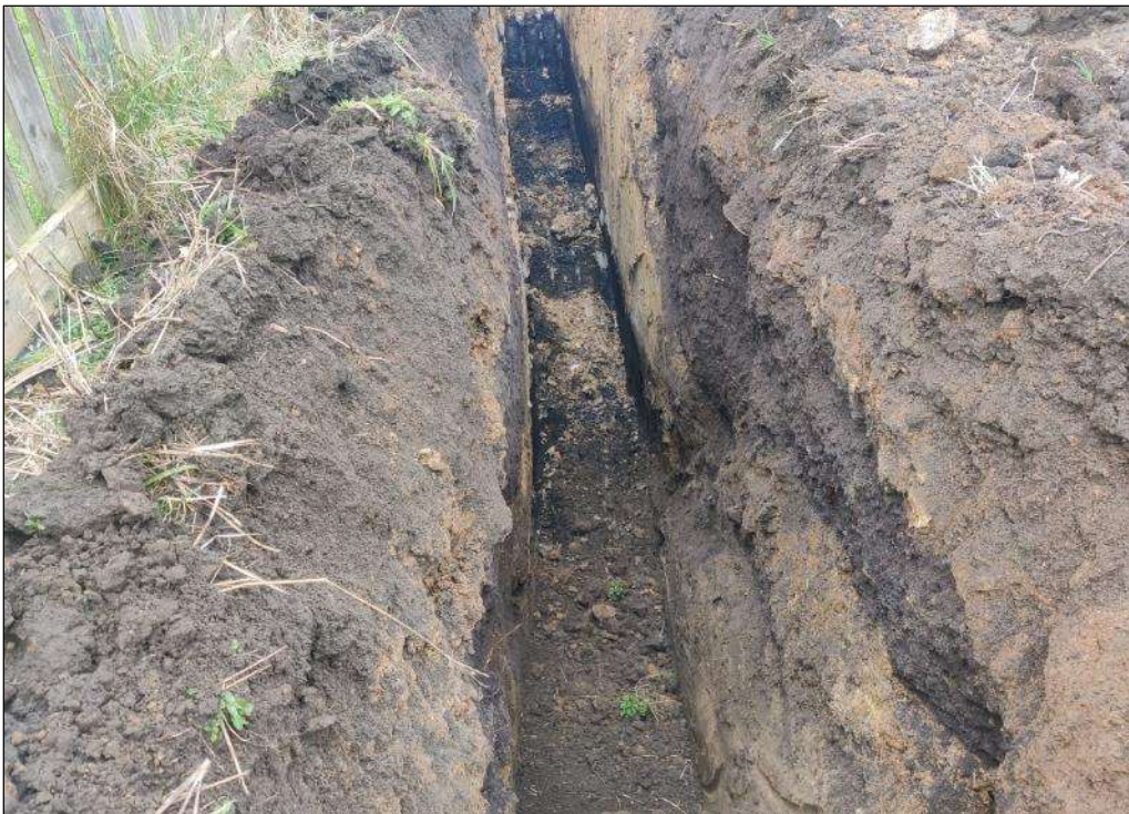
Photo 4: TP01 – Dark coloured infill material within the natural light brown strata.
