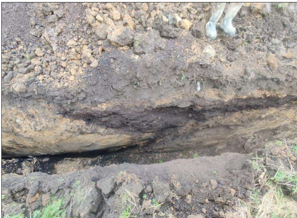
Photo 2: TP01 – Dark coloured infill material within the natural light brown strata.
