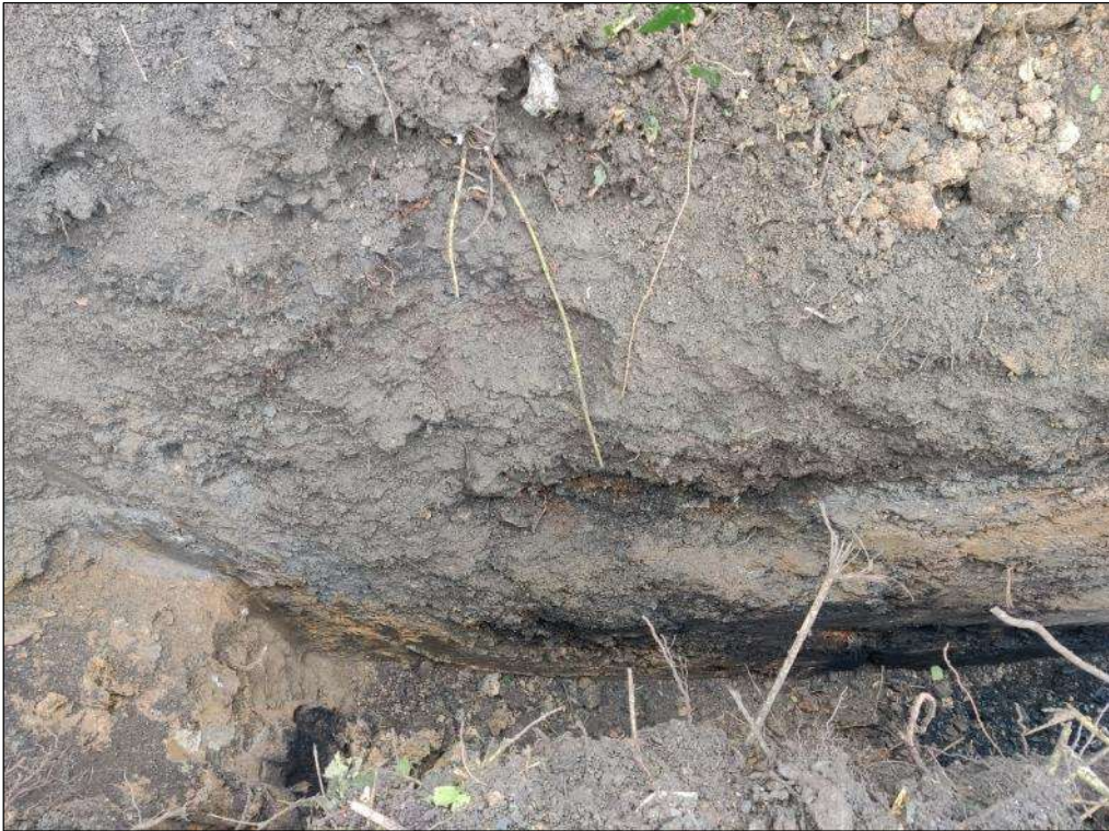
Photo 7: TP03 – Darker coloured backfill material with fragments of brick (adit 16) within the light brown natural strata.
