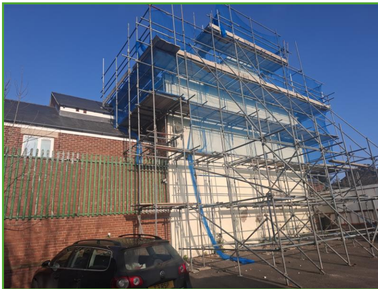
Photo 1: View of southern gable end of Building B1 (former Fitzwilliam Public House)
