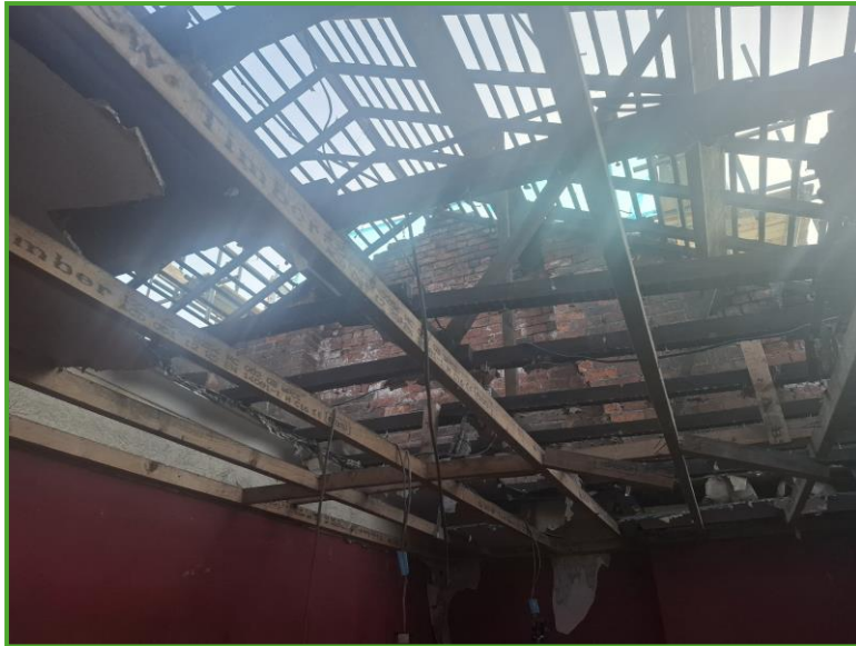
Photo 2: View of Building B1 southern gable wall with both chimneys removed and clay roof tiles.
