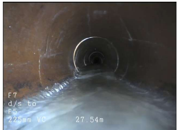
Photo: 8_13A 27.55m, Crack, circumferential, from 7 to 3 o'clock
