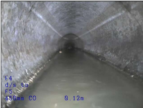
Photo: 5_3A, 00:00:10 0.12m, Crack, circumferential, from 9 to 4 o'clock
