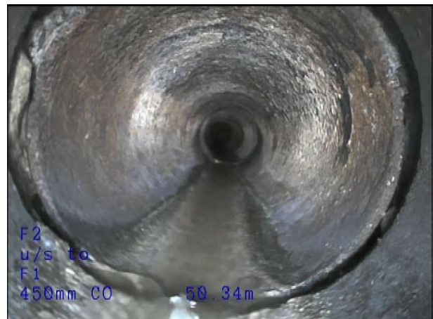
Photo: 2_6A 50.34m, Open joint, medium Remarks: Backfill visible
