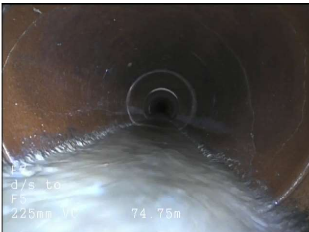
Photo: 8_31A 74.75m, Crack, circumferential, from 7 to 5 o'clock
