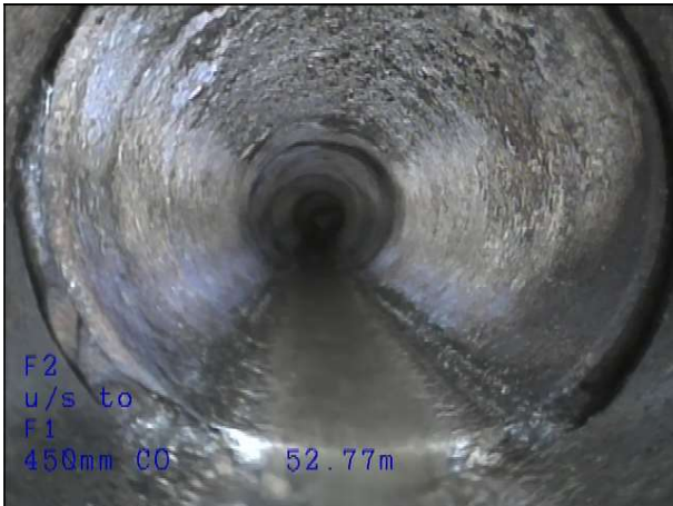
Photo: 2_7A 52.77m, Open joint, medium
