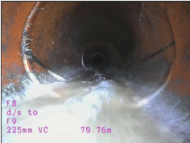
Photo: 12_19A 70.76m, Fracture, longitudinal at joint, at 2 o'clock
