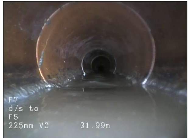
Photo: 8_18A 31.99m, Crack, circumferential at joint, from 8 to 11 o'clock
