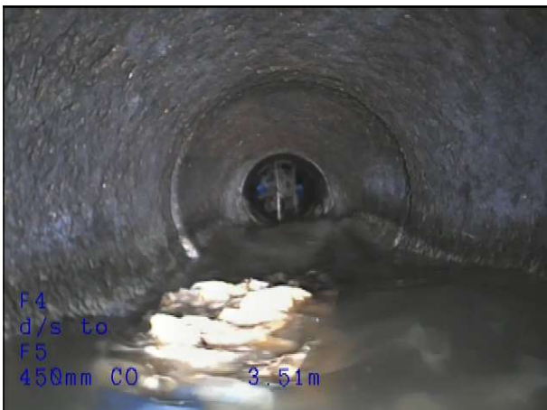
Photo: 5_6A 3.51m, Settled deposits, coarse, 20% cross-sectional area loss
