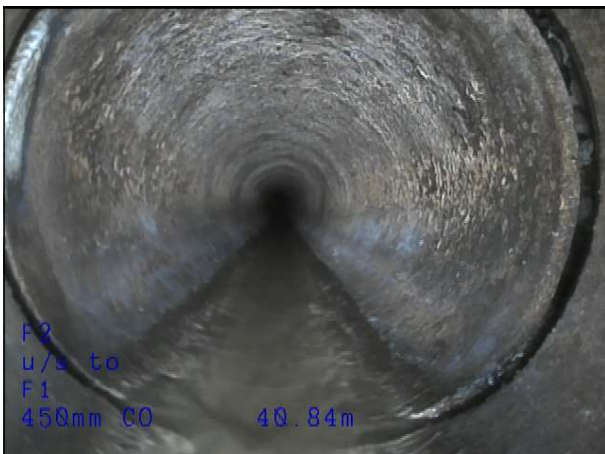
Photo: 2_5A 40.84m, Open joint, medium Remarks: Backfill visible
