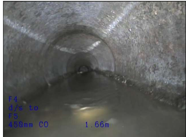
Photo: 5_4A 1.67m, Settled deposits, coarse, 10% cross-sectional area loss, Start
