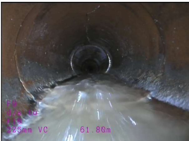
Photo: 14_11A 61.8m, Crack, longitudinal at joint, at 12 o'clock
