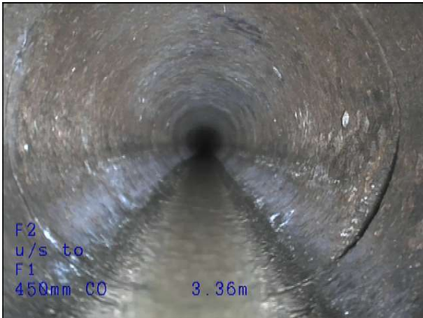
Photo: 2_3A 3.36m, Surface damage, spalling, from 3 to 5 o'clock Remarks: At joint
