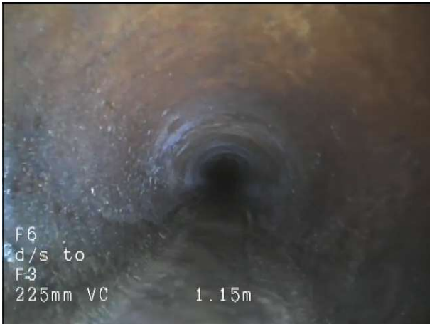
Photo: 7_4A 0m, Point repair, localised lining, from 12 to 12 o'clock, Start Remarks: Cured in place lining installed
