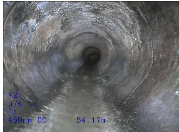
Photo: 2_8A 54.17m, Fracture, circumferential, from 12 to 12 o'clock
