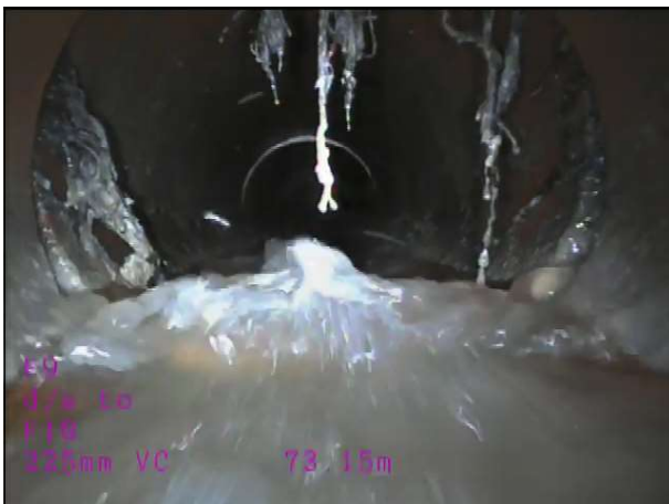
Photo: 14_16A 73.15m, Roots, mass at joint, 10% cross-sectional area loss
