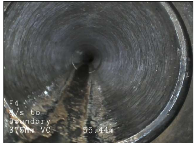
Photo: 6_4A 55.44m, Open joint, medium
