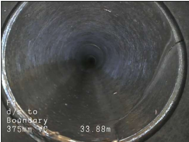
Photo: 6_3A 33.88m, Fracture, circumferential at joint, from 2 to 5 o'clock
