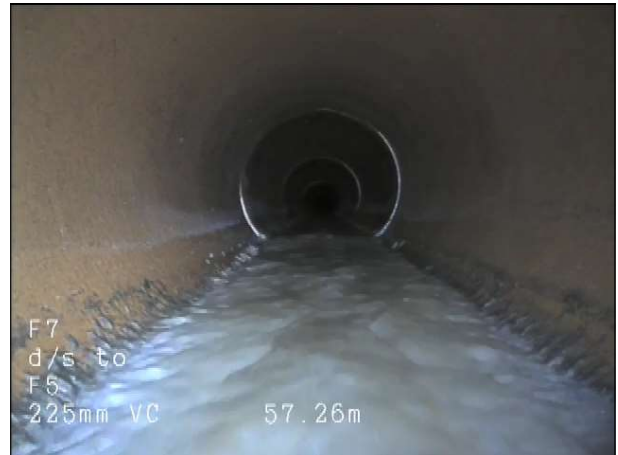
Photo: 8_28A 56.57m, Crack, circumferential at joint, from 1 to 5 o'clock
