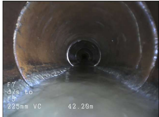
Photo: 8_23A 42.2m, Fracture, circumferential at joint, from 1 to 5 o'clock
