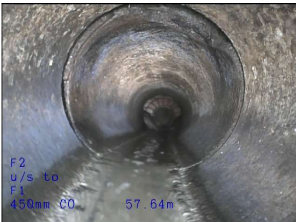
Photo: 2_9A 57.67m, Hole in drain/ sewer at joint, from 11 to 2 o'clock Remarks: Pipework missing
