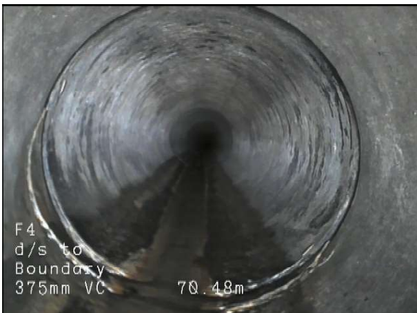
Photo: 6_6A 70.48m, Fracture, circumferential at joint, from 4 to 9 o'clock
