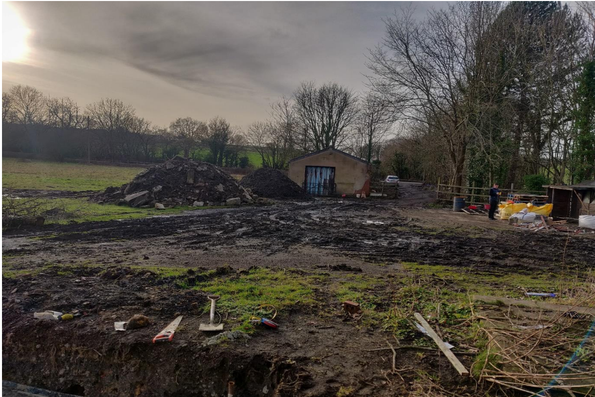
VIEW WITH SITE IN FOREGROUND LOOKING WEST TOWARDS EXISTING STABLES (works to convert to dwelling in progress).
